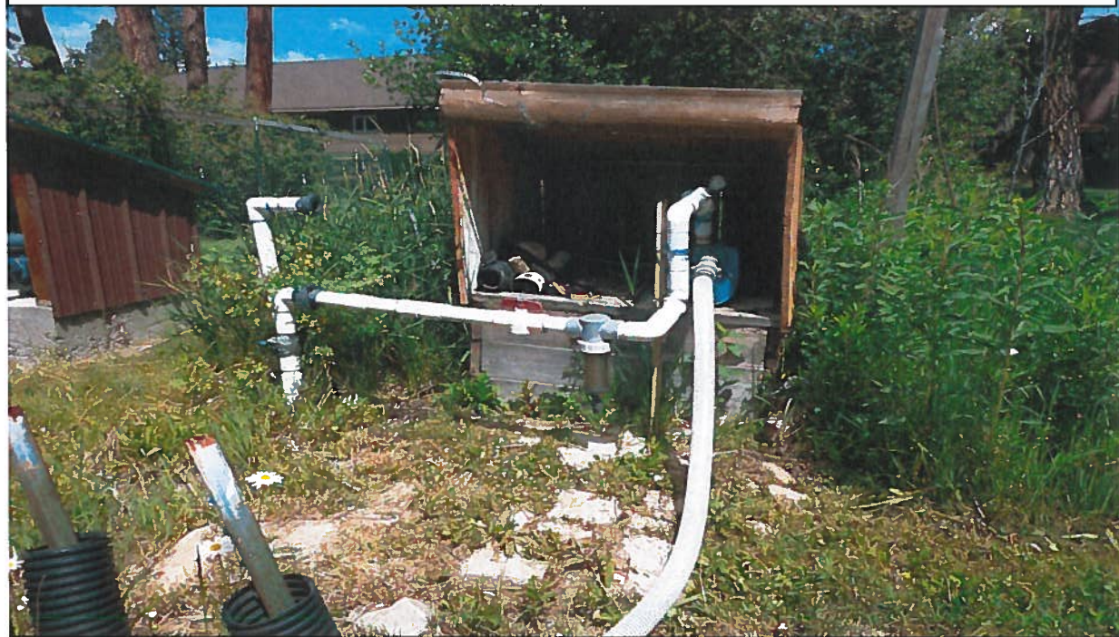
View northerly of the 2-hp centrifugal pump, 2" flexible hose suction line, 2" PVC discharge main line, and enclosure.
