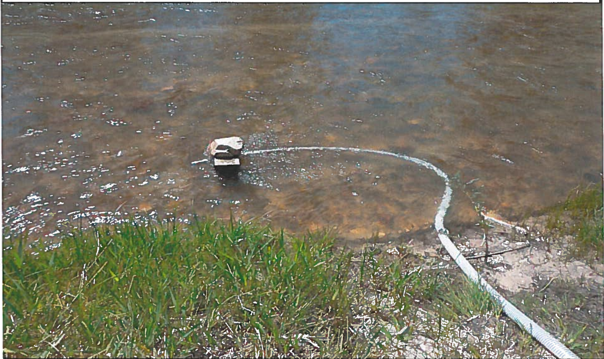
Point of Diversion: View southerly of the screened intake and the 2" flexible hose suction line near the north bank of the Middle Fork of the Payette River.
