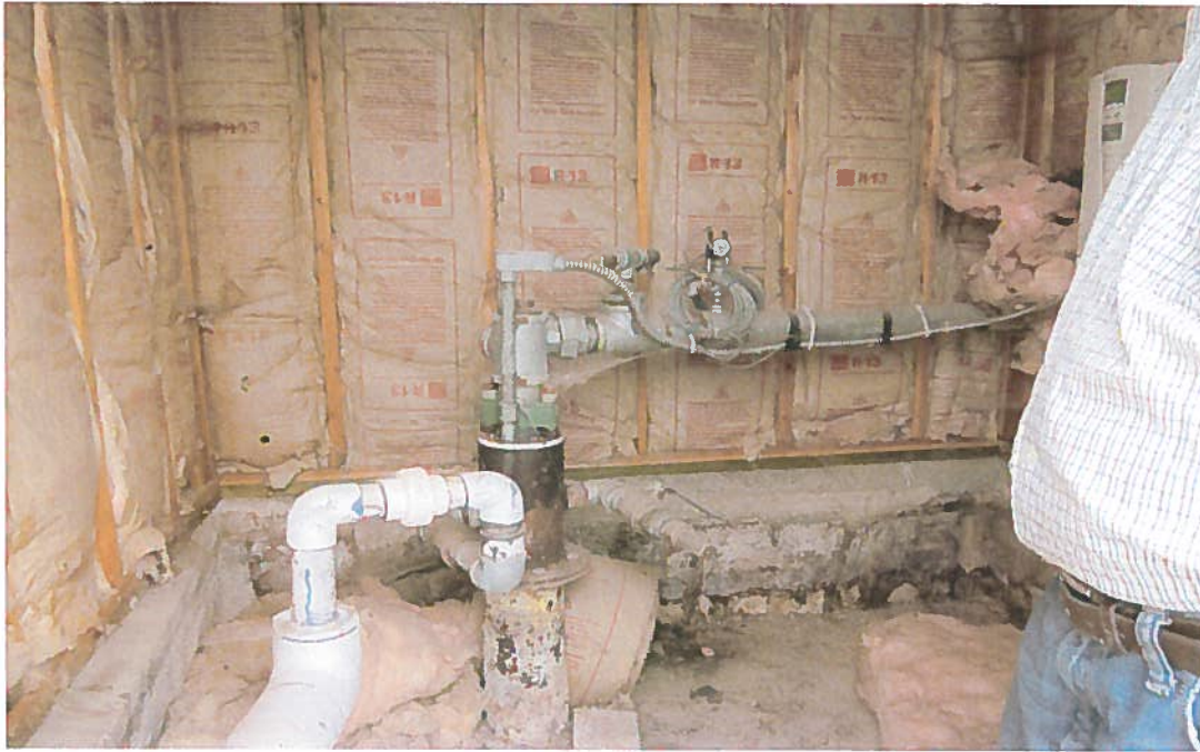
The old artesian well seen here, located in the pump house, is one of the PODs for fire protection.
