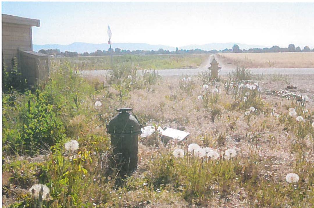
The newer well and second POD is seen front center. The pump house is seen in the left. The wells are plumbed to the hydrant seen in background .
