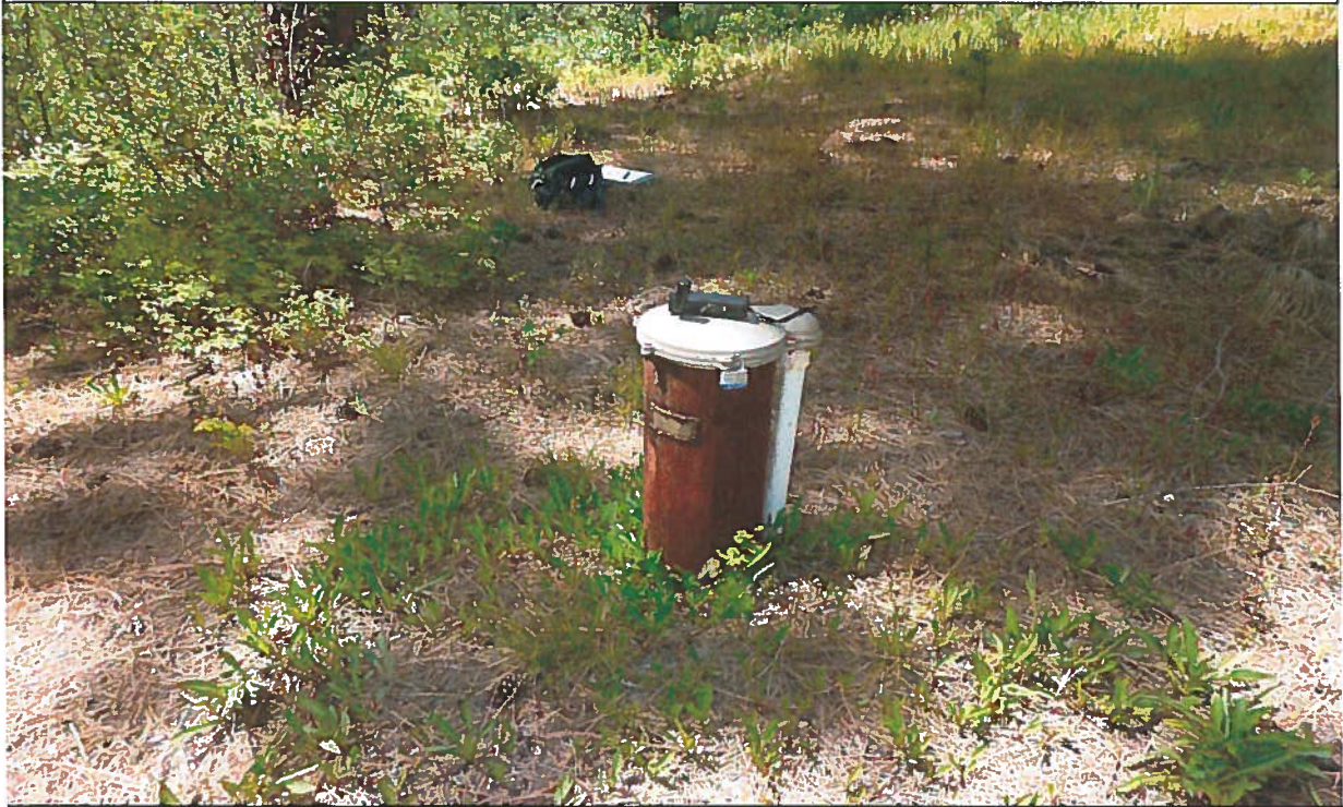
Point of Diversion: View westerly of the ground water well located on Lot 27, Shiloh Ranch Estates.
