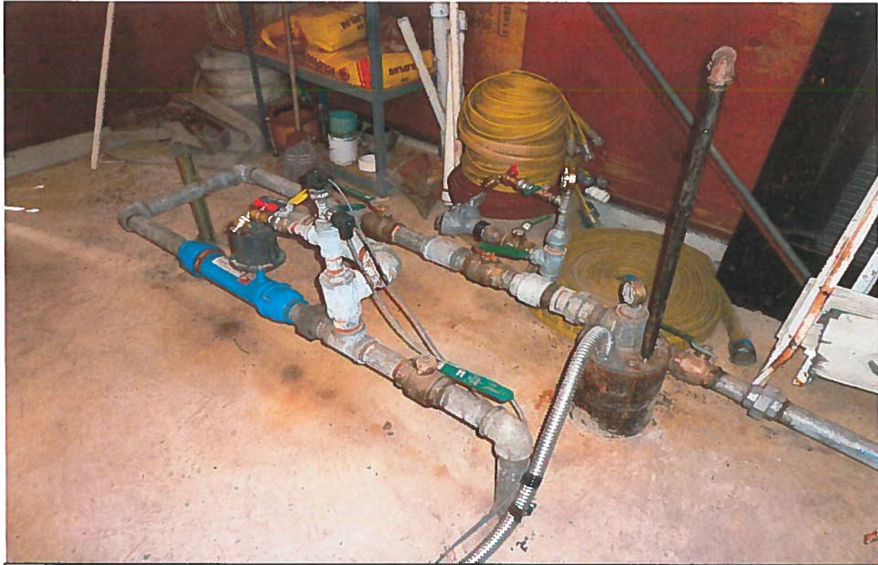
Point of Diversion: View of ground water well in well/pump house located on Lot 27, Shiloh Ranch Estates.
