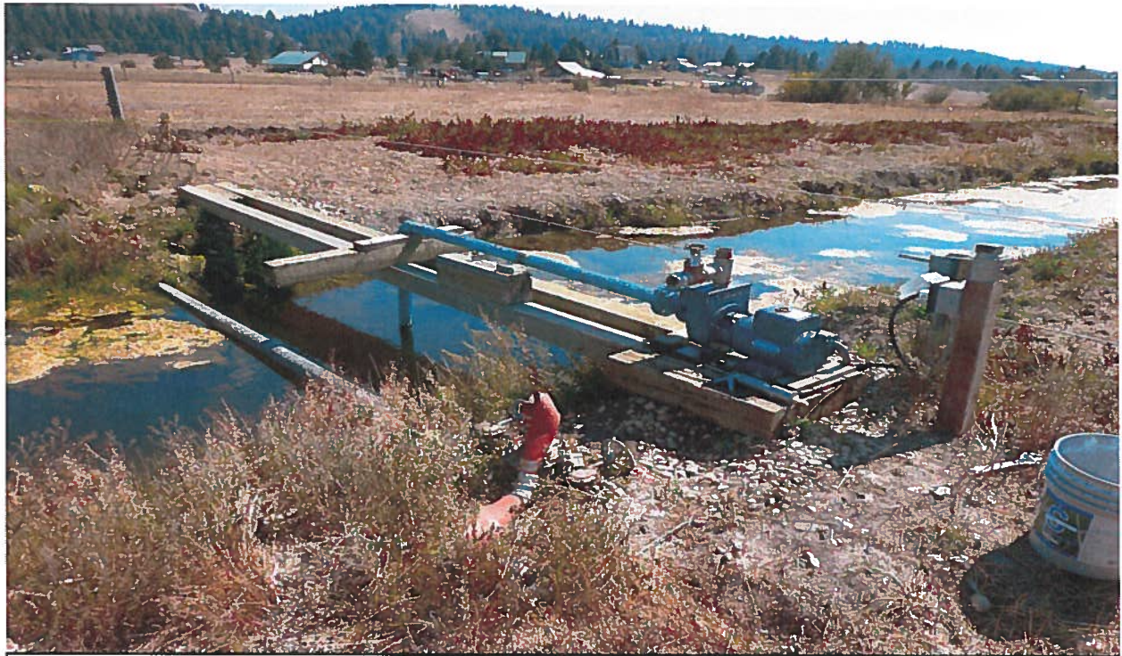
View southeasterly of the irrigation/aesthetic storage pond and a 5-hp Berkley irrigation centrifugal pump which diverts water from the storage pond through a 3" suction line. The irrigation pump discharges water through a 4" flexible hose to the 4" Schedule 40 irrigation main line.
