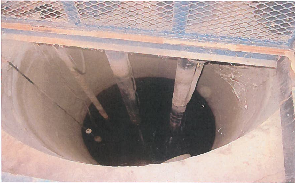
Sump inside the pump house.
