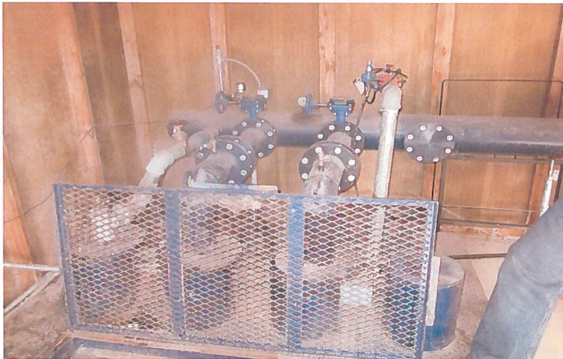
Piping in the pump house that conveys the co-mingled shallow ground water and Settlers irrigation District surface water to the subdivision.
