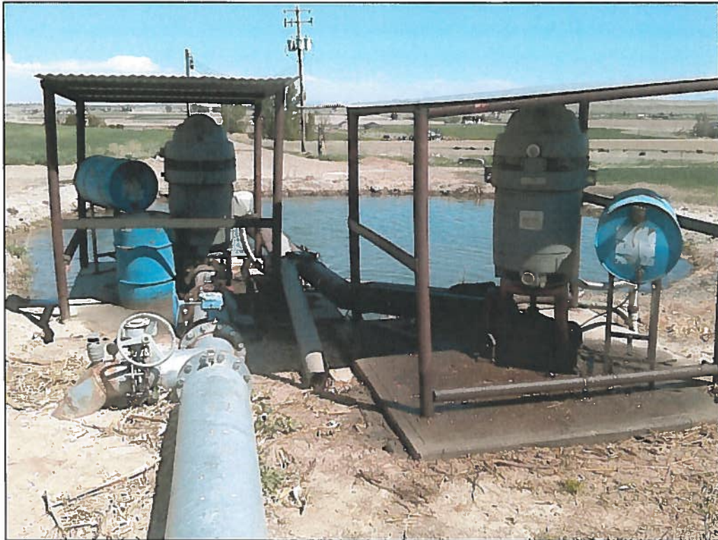
Figure 3: East well (on right) and booster pump. Both are 125-hp turbines.
