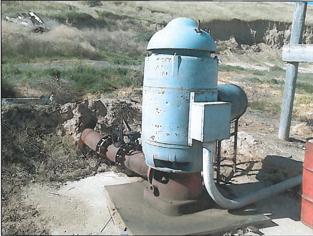
Figure 1: North Well is 200-hp vertical turbine.
