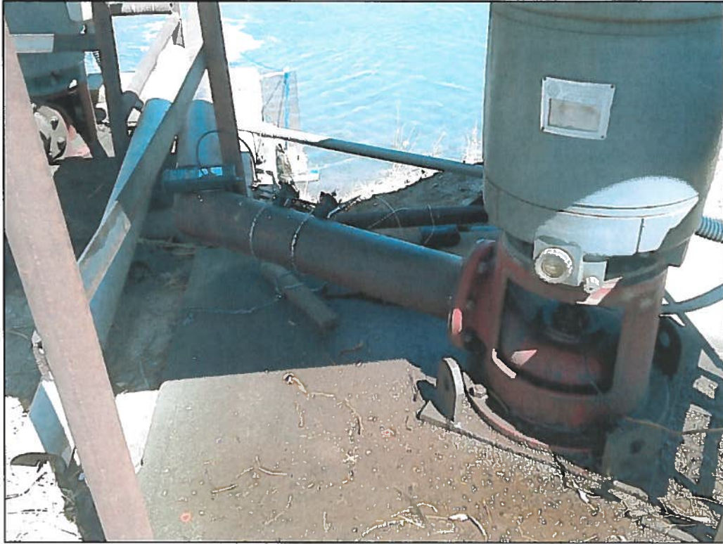
Figure 5: East well showing location of ultrasonic flowmeter with measured discharge of 735 gpm.
