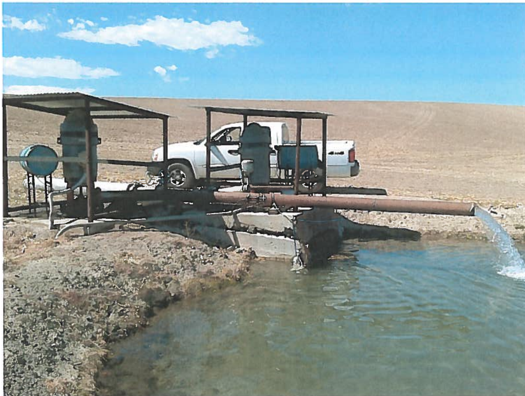
Figure 4: East well (on left) and booster (center). Ultrasonic meter did not obtain adequate signal at the location shown.
