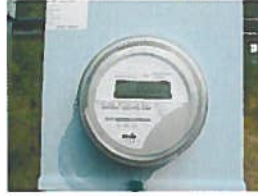
POWER WELL #7 .JPG
