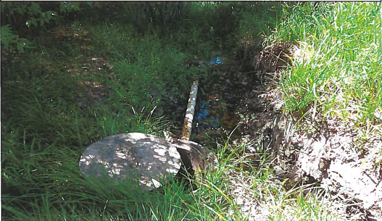
Point of Diversion: View southwesterly of the 3' diameter concrete spring box and the 4" PVC perforated pipe supply line in a spring. Spring water is discharged through 2" steel pipe to a 500-gallon fiberglass buried water storage tank.
