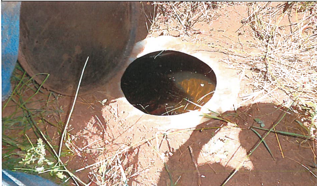
View westerly of the buried 500-gallon fiberglass storage tank. Spring water is discharged through 2" steel pipe to a watering trough located within a corral. The 500-gallon water storage tank contains a 3" steel overflow pipe which daylights to a drainage swale east of the water storage tank.
