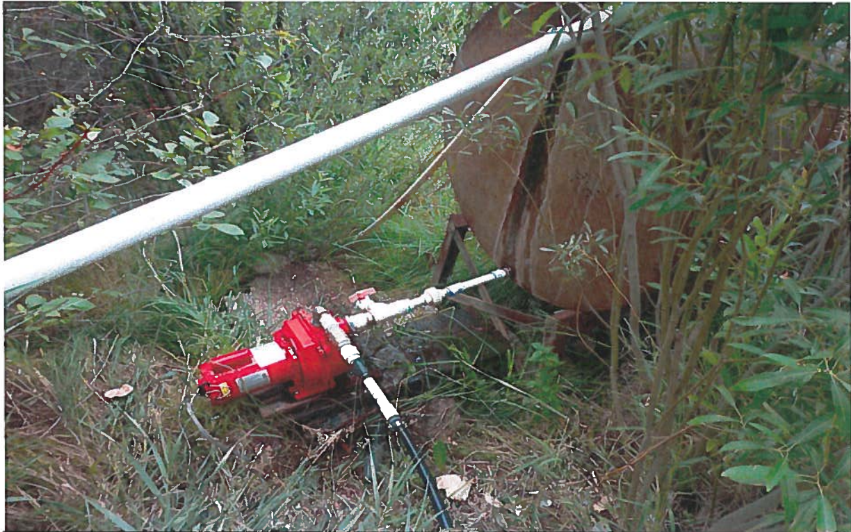
View of the 1" PVC supply line discharging to the top of the 300-gallon steel water storage tank, and a \frac{3}{4} -hp centrifugal pump with a \frac{3}{4} " PVC discharge line. Water is pumped from the water storage tank to irrigate a garden area and fruit trees.
