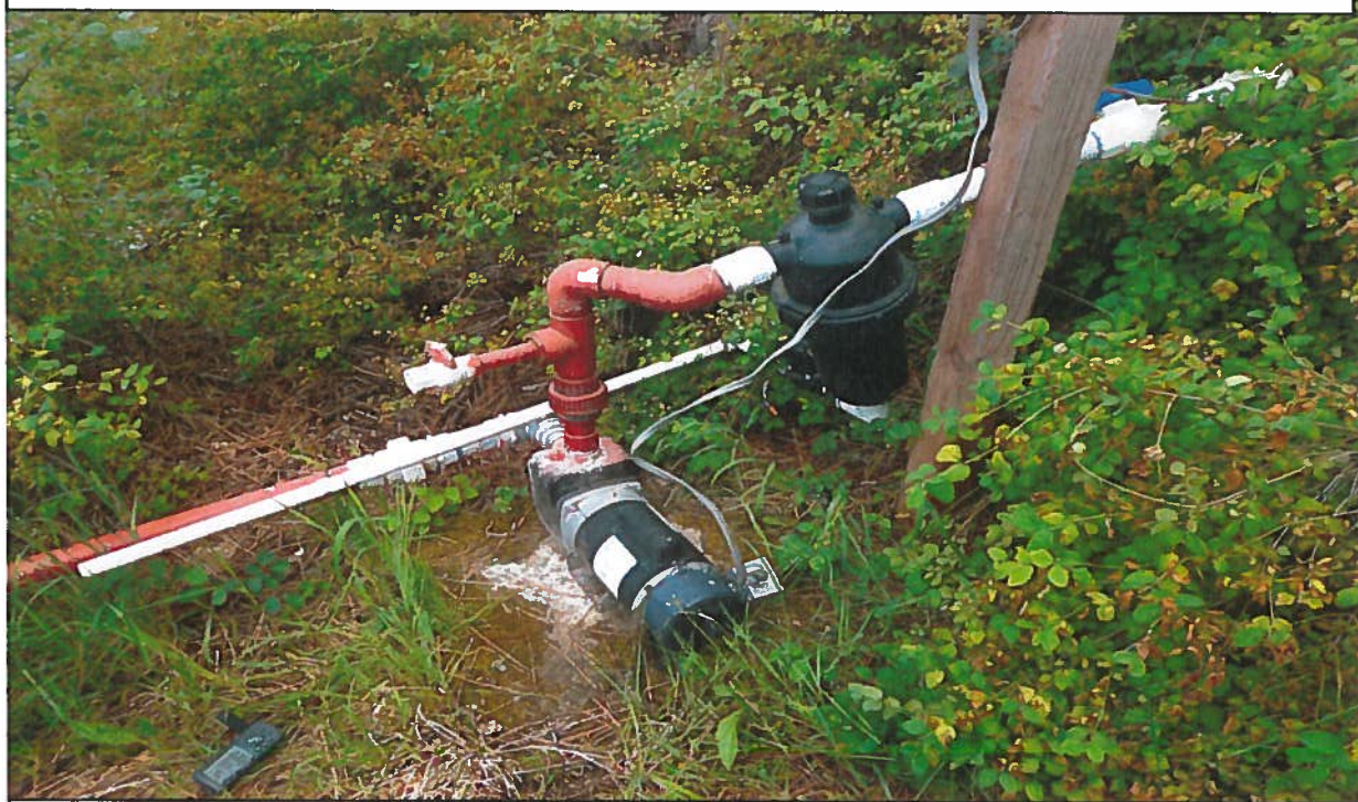
View of a 2-hp centrifugal pump and the 2" PVC irrigation supply line.
