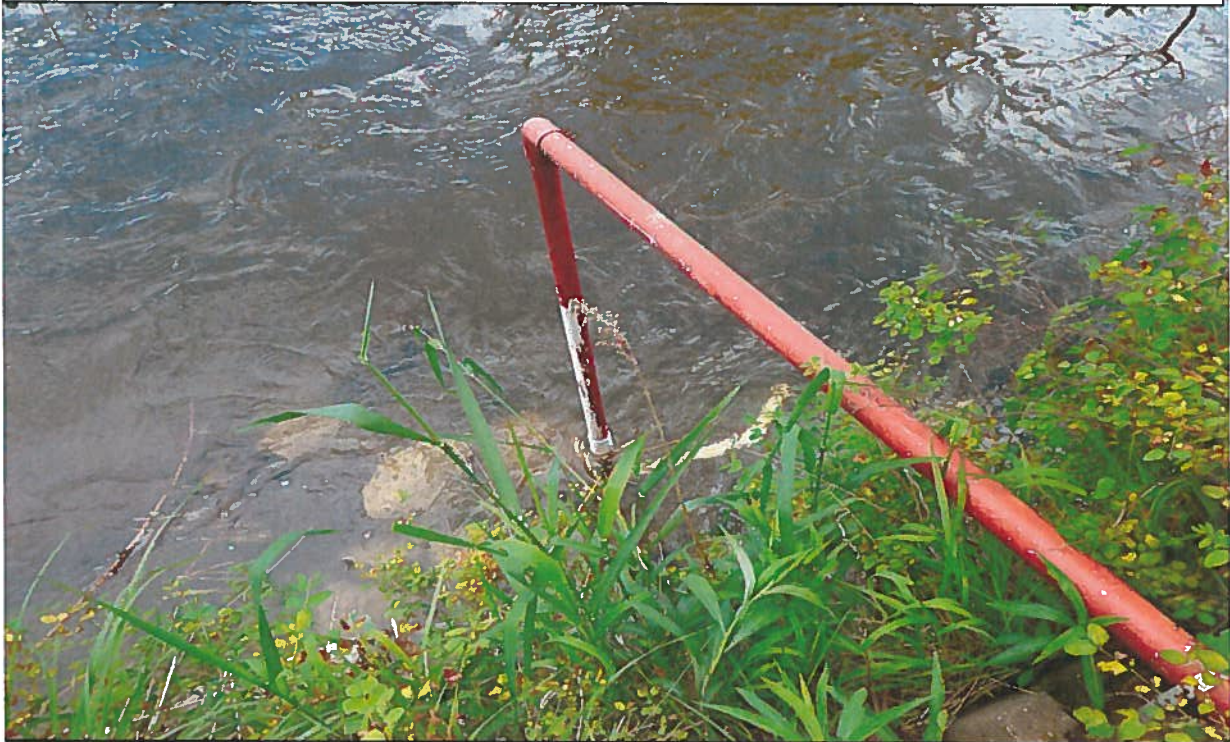
Point of Diversion: View of the 2" PVC suction line located near the southerly bank of the Middle Fork of the Payette River.
