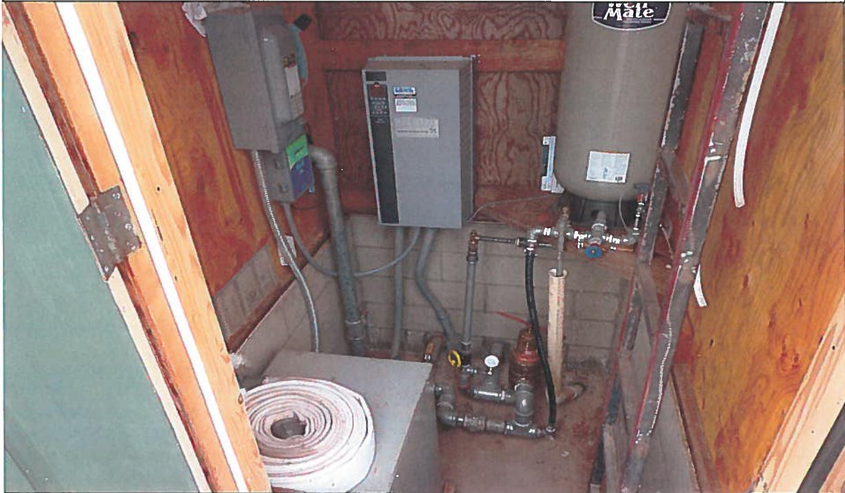
Point of Diversion: View inside of well house of the 2 1/2" galvanized well discharge piping and the Danfoss VLT Aqua Drive VFD.
