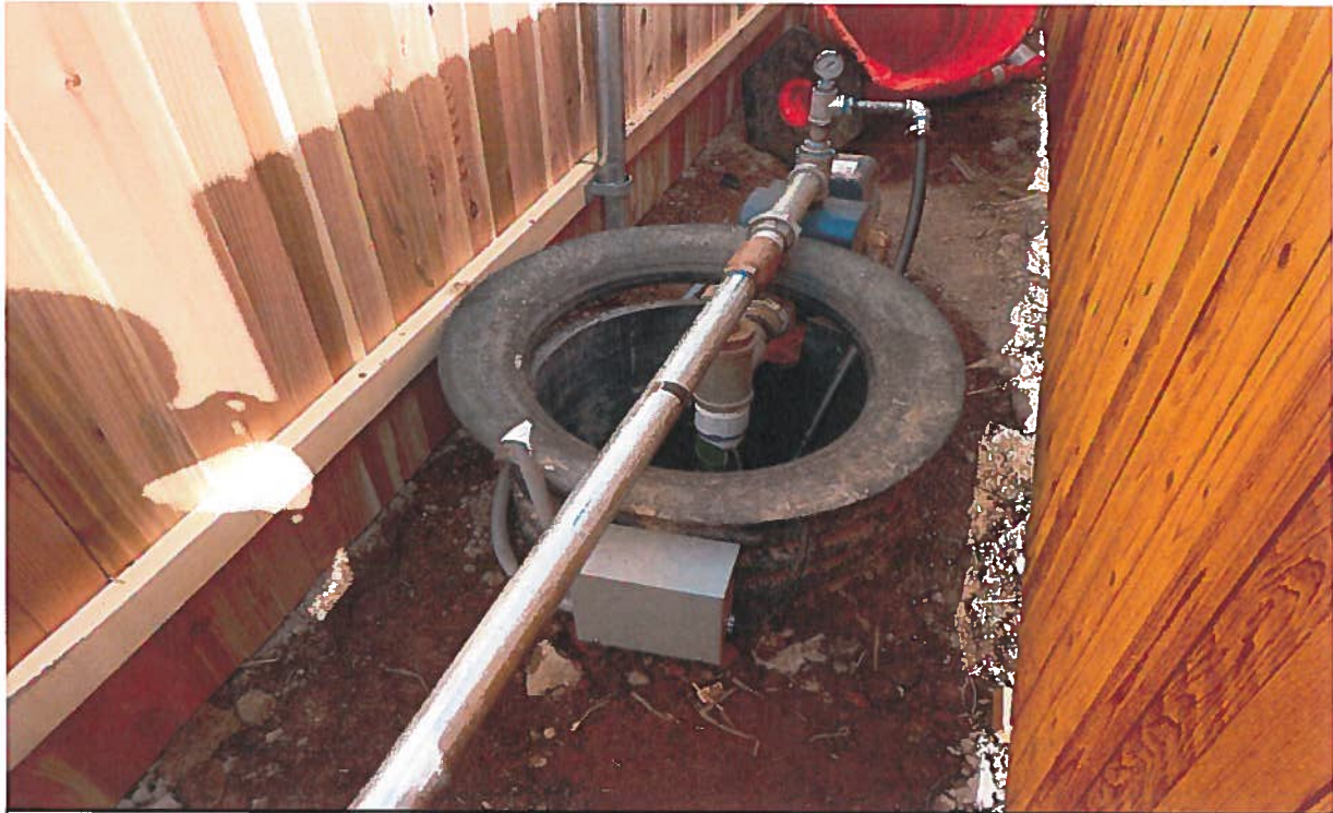
View northerly of the 2' diameter sump/vault and the 2" Schedule 40 steel discharge line. A 5-hp submersible pump diverts surface water from the sump/vault through a 4" suction line. Surface water is discharged through the 2" Schedule 40 steel supply line to the Aspen Hill Apartments pressurized irrigation system.
