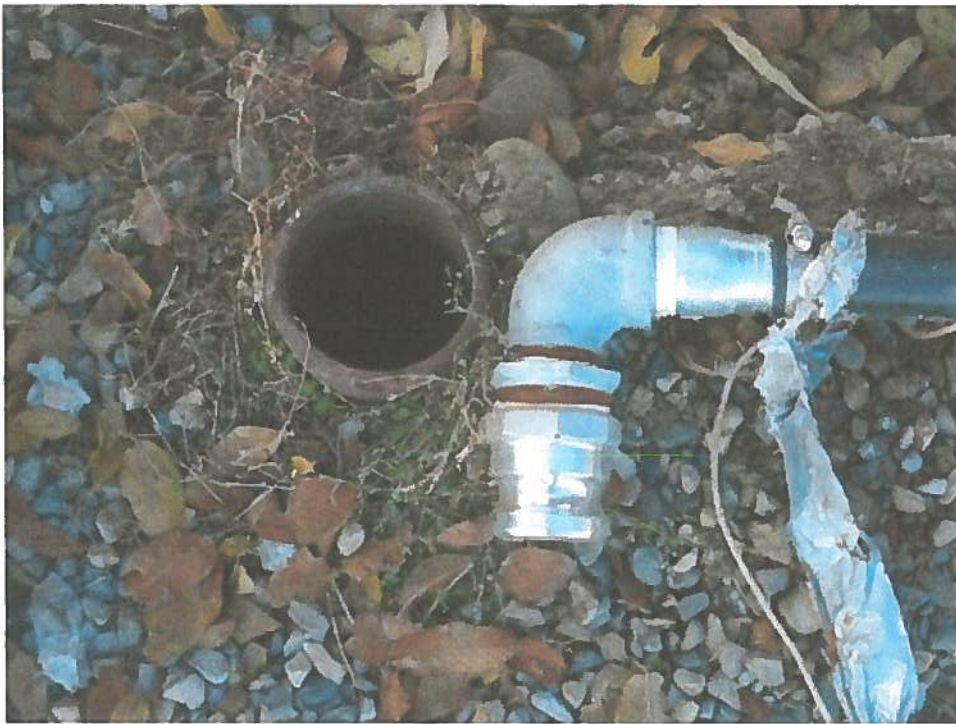
Point of Diversion / Pump adapter (2" Line)
