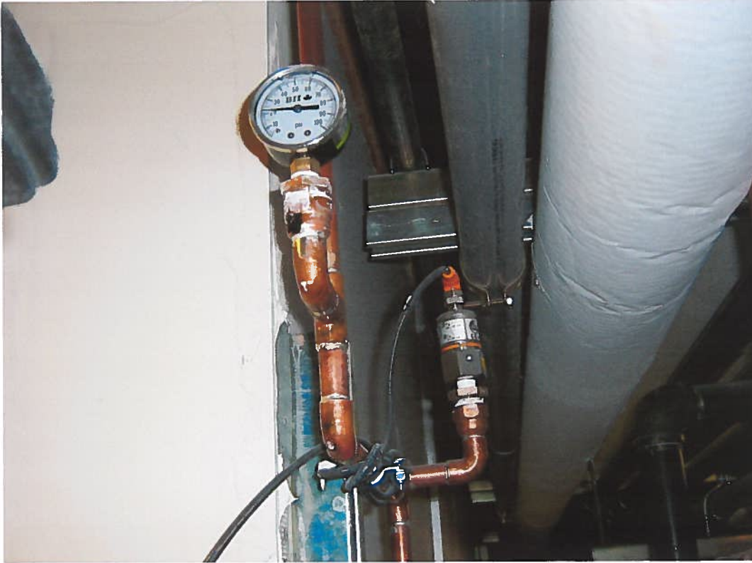
Inlet pressure and sensor for VFD
