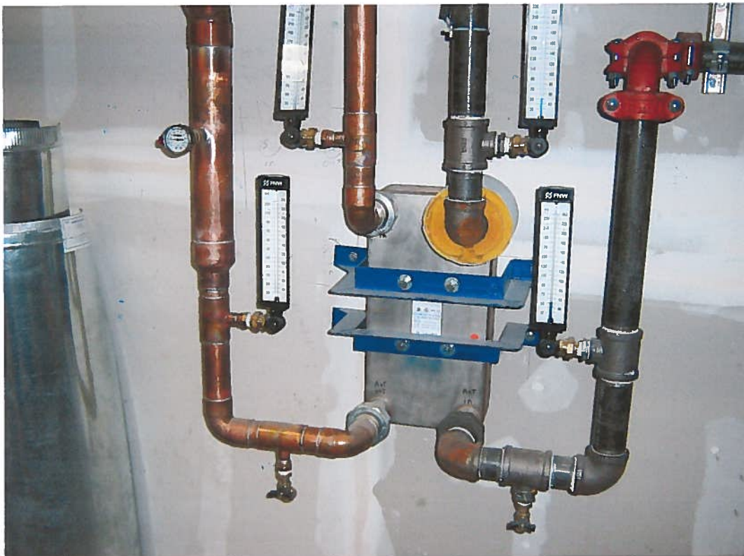
Heat exchanger for cooling
