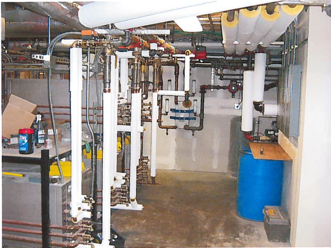
Piping at rear of heat pumps
