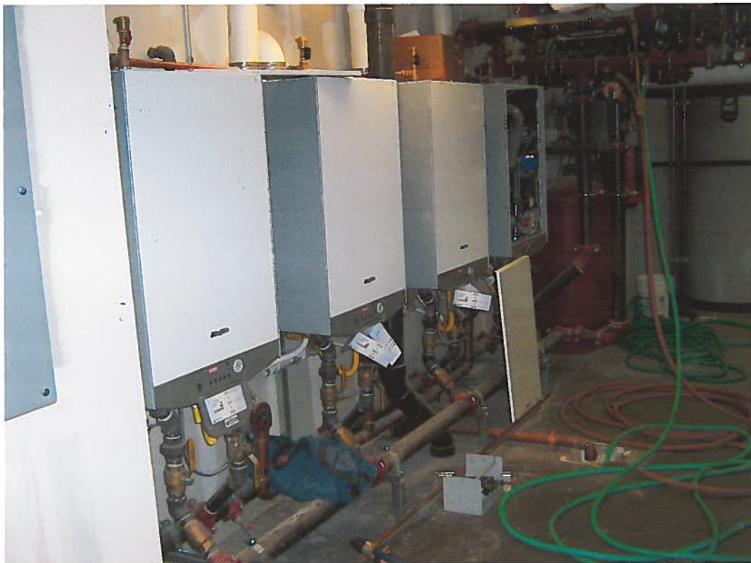
Supplemental natural gas-fired boilers
