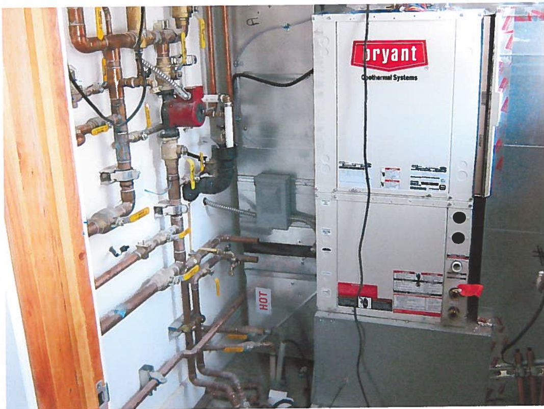
Heat exchanger system for barn
