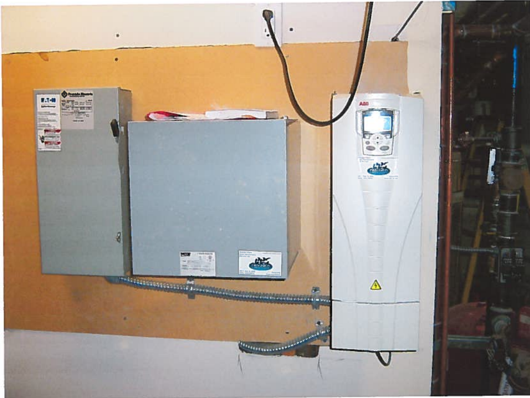
Pump controller – 3 phase converter and VFD
