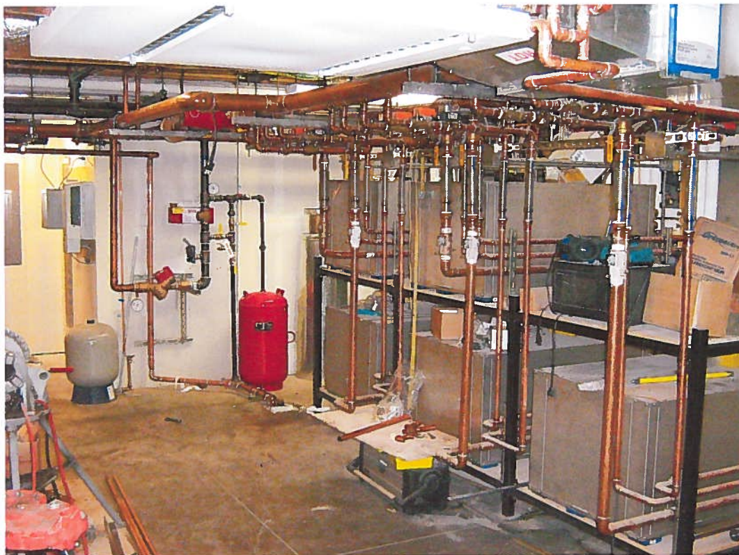
Piping in dedicated utility room showing five heat pumps, pump controller at extreme left
