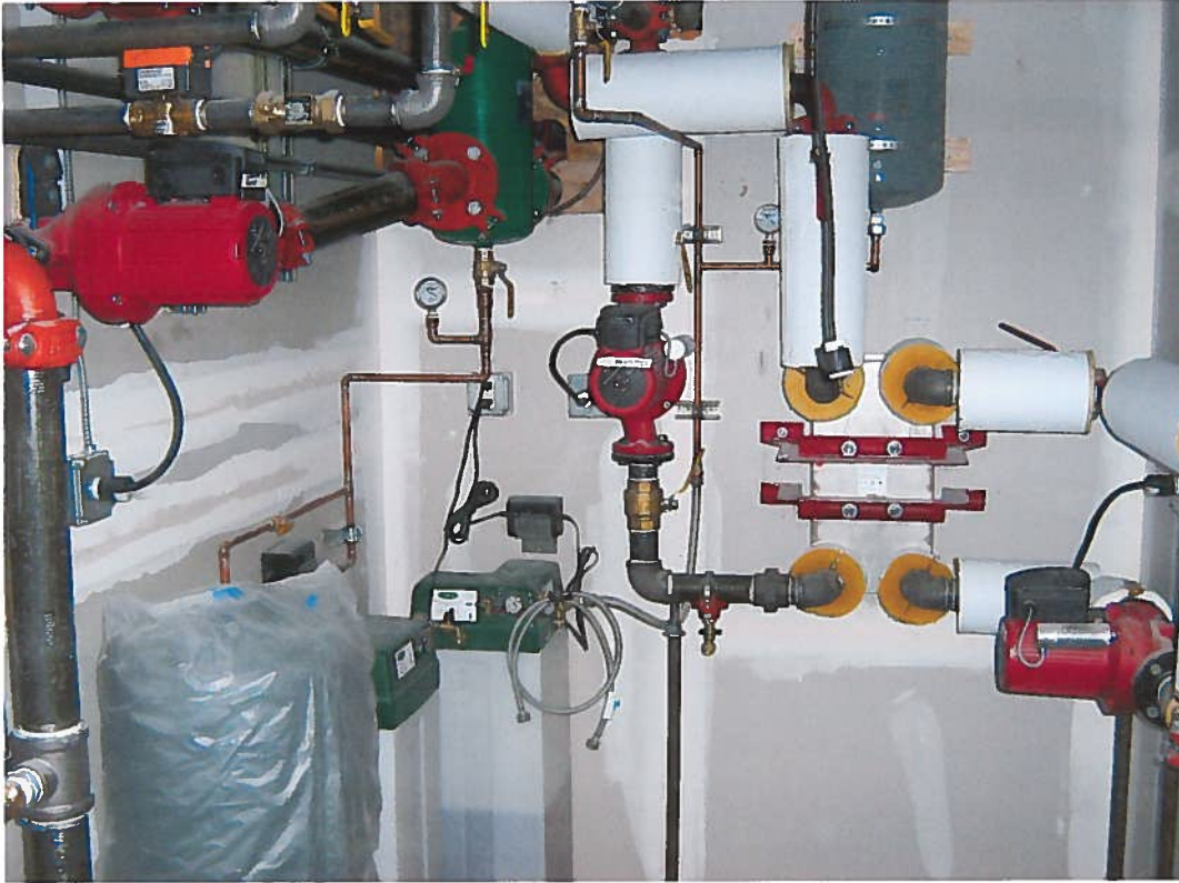
Heat exchangers and booster pumps
