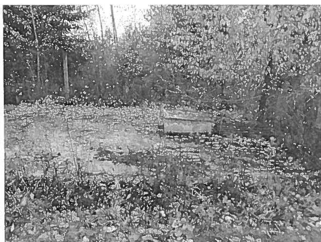
30,000-gallon concrete grade reservoir
