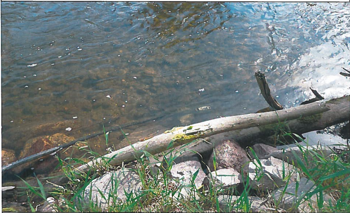
Point of Diversion: View northerly of the screened 1 1/2" PVC suction line near the southerly bank of the Middle Fork of the Payette River.
