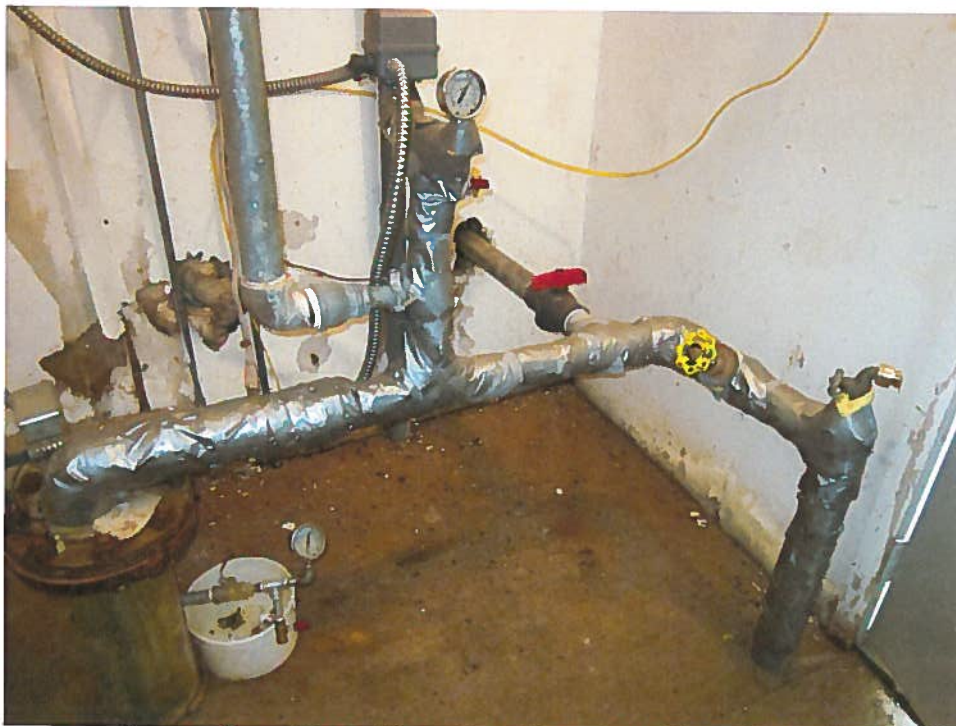
Inside the booster pump house
