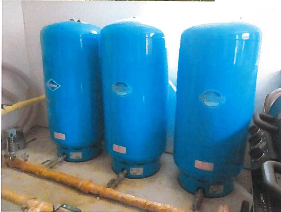
Tanks inside the new pump house
