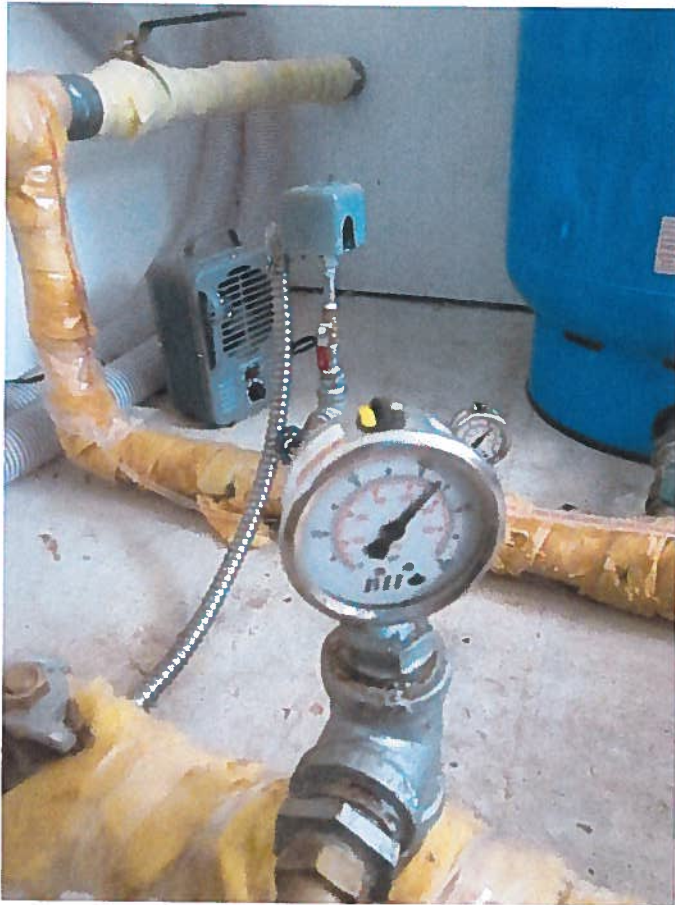
Gage in pump house
