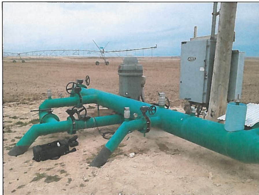
Figure 2: Measured flow was diverted through one mainline to the pond.
