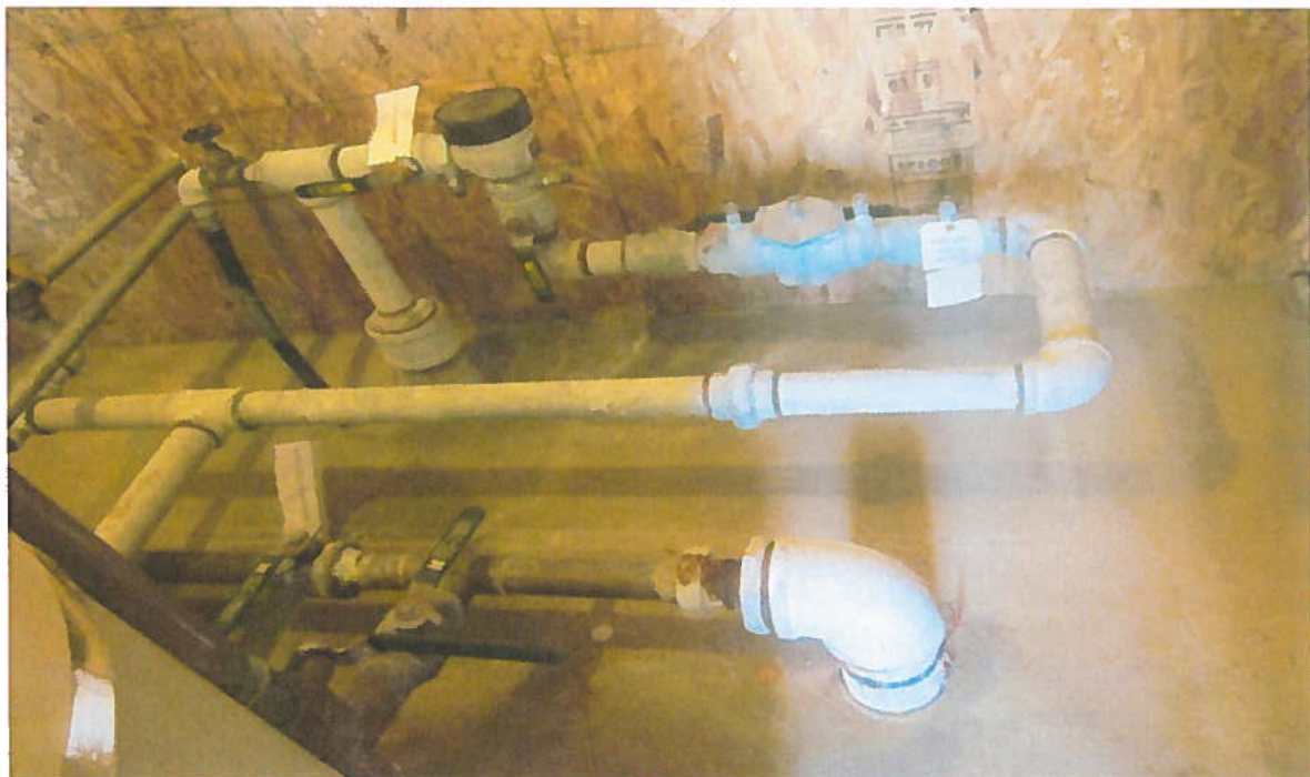
Piping in front plumbed to sprinkler irrigation system. Domestic system piping seen in background.
