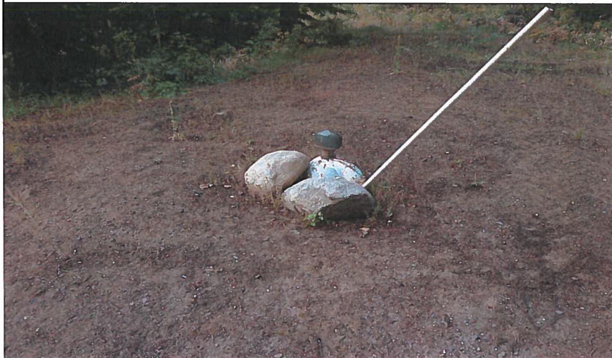
Point of Diversion: View of the ground water well which serves eight homes within the Mile High Estates Subdivision. The well is located easterly of a log pump house.
