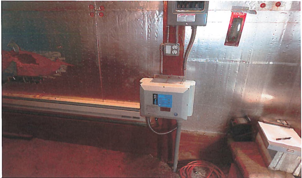
View inside the pump house of a Franklin VSD Subdrive 300 Variable Frequency Drive system which controls the water system operations.
