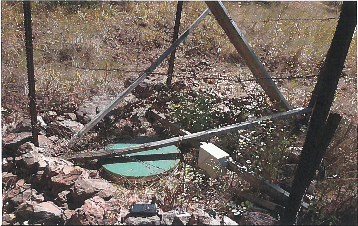
View southeasterly of the 1,000-gallon pump vault located near the spring box. A submersible pump diverts water through approximately 900 lineal feet of 1 1/4" PVC pipe to a pressure tank located in a shop near the home.
