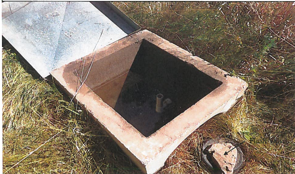
Point of Diversion: View inside of spring box and the 1 1/4" PVC pipe which discharges water to a 1,000-gallon buried pump vault. The valve box contains a 1 1/4" valve to allow periodic flushing of the spring box.
