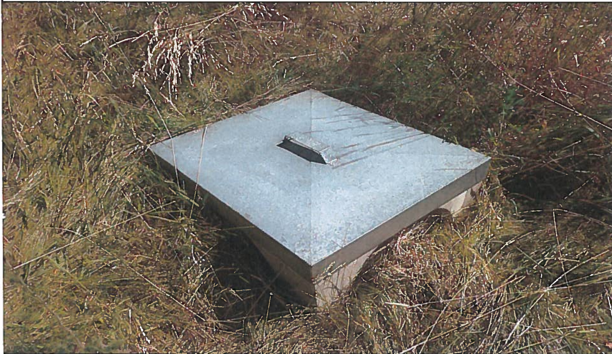
Point of Diversion: View of spring box. Spring water is discharged from the spring box through 1 1/4" PVC pipe to a 1,000-gallon buried pump vault.
