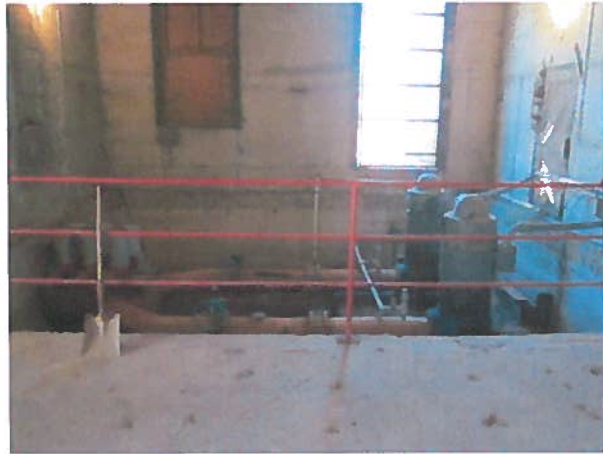
Two 200 hp pumps in pumphouse
