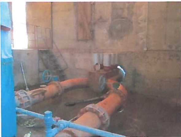
Manifold of pumps leaving the pumphouse
