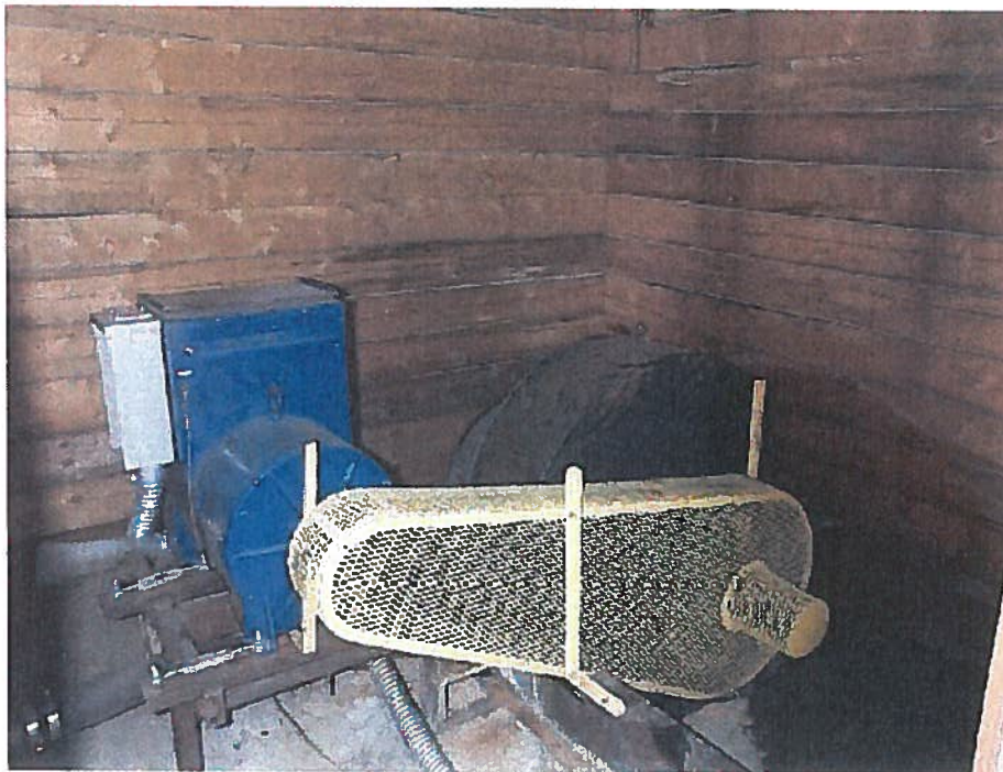
4. Turbine and generator with new protective housing.
