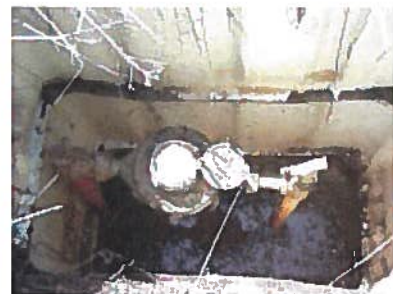
Vault with flow meter and sample tap
