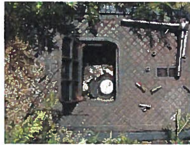
Vault with flow meter
