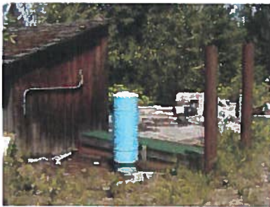
Pump house and main reservoir
