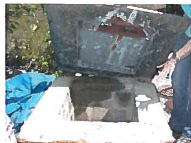
Access hatch – needs gasket
