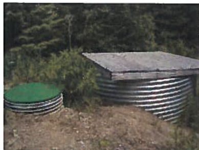
Reservoir lid and valve pit
