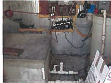
Reservoir access and chlorinator
