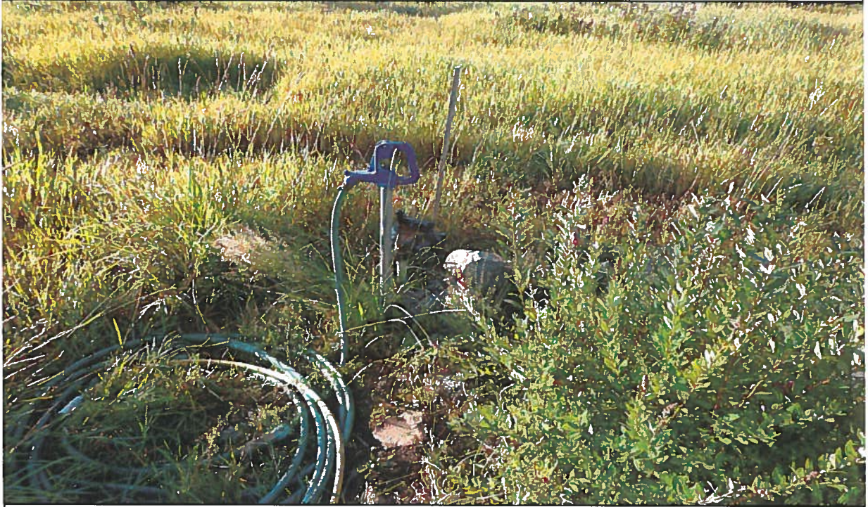
Point of Diversion: View of ground water well located near a small pump enclosure.
