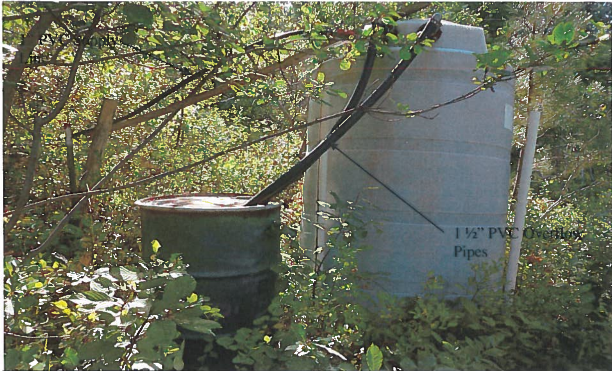
View of the 1" PVC supply line discharging to the top of the 500-gallon fiberglass water storage tank. Two 1 1/2" PVC overflow pipes from the water storage tank discharge water to a 50-gallon drum. Water collected in the 50-gallon drum is discharged in 1" PVC pipe to a 5-gallon bucket in the Unnamed Stream. A 1 1/2" PVC discharge pipe from the 5-gallon bucket discharges to a stock tank.
