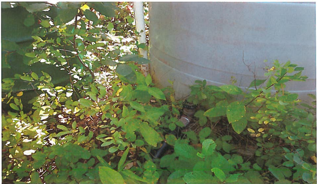
View of the 1 1/2" PVC pipe supply line at the bottom of the 500-gallon water storage tank. A hand operated gate valve controls the flow to the frost-free hydrant near the home.
