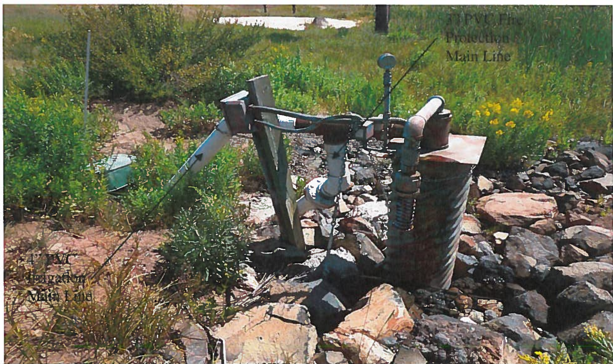
Point of Diversion: View easterly of a 15" perforated CMP stand pipe in which contains a 10-hp submersible pump. Water is discharged through a 4" PVC irrigation main line to operate the irrigation system. The 3" PVC fire protection main line to the fire hydrant 'tees' off the 4" irrigation discharge pipe.
