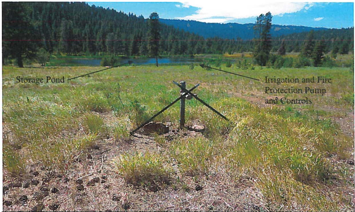
View southwesterly of the fire hydrant for fire protection. The fire hydrant is constructed of 3" steel pipe with 3" and 1 1/2" nozzles for hose attachment to fight a fire or for fill the holding tanks in fire trucks. A 10-hp pump irrigation and fire protection pump diverts water from the storage pond to the fire hydrant through a 3" main line.
