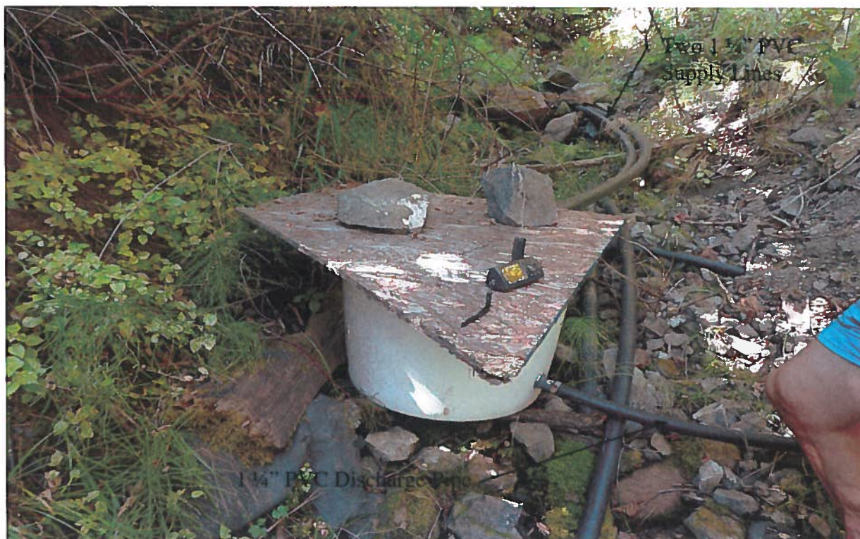
Point of Diversion: View westerly of a 3' diameter by 2' deep water storage tank. Water is diverted from an Unnamed Stream through two 1 1/4" PVC pipes. Water is discharged from the water storage tank through 1 1/4" PVC to the right holder's irrigation system.
