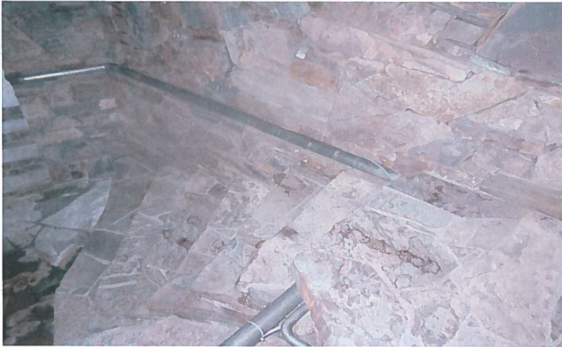
Steel piping from spring to bottling plant.
