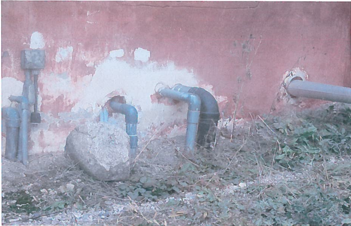
Piping from the springs to the bottling plant. Electrical box and conduit seen in the left of the picture, the three pipes from the three springs seen center.
