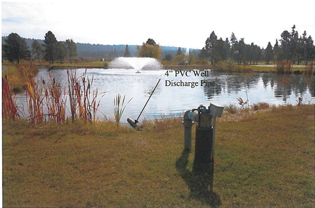
Point of Diversion: View easterly of the ground water well located near the irrigation/recreation storage pond which diverts water to the pump station wet well for irrigation of the McCall Golf Course. The ground water well's 4" PVC discharge line is shown extending into the storage pond.
