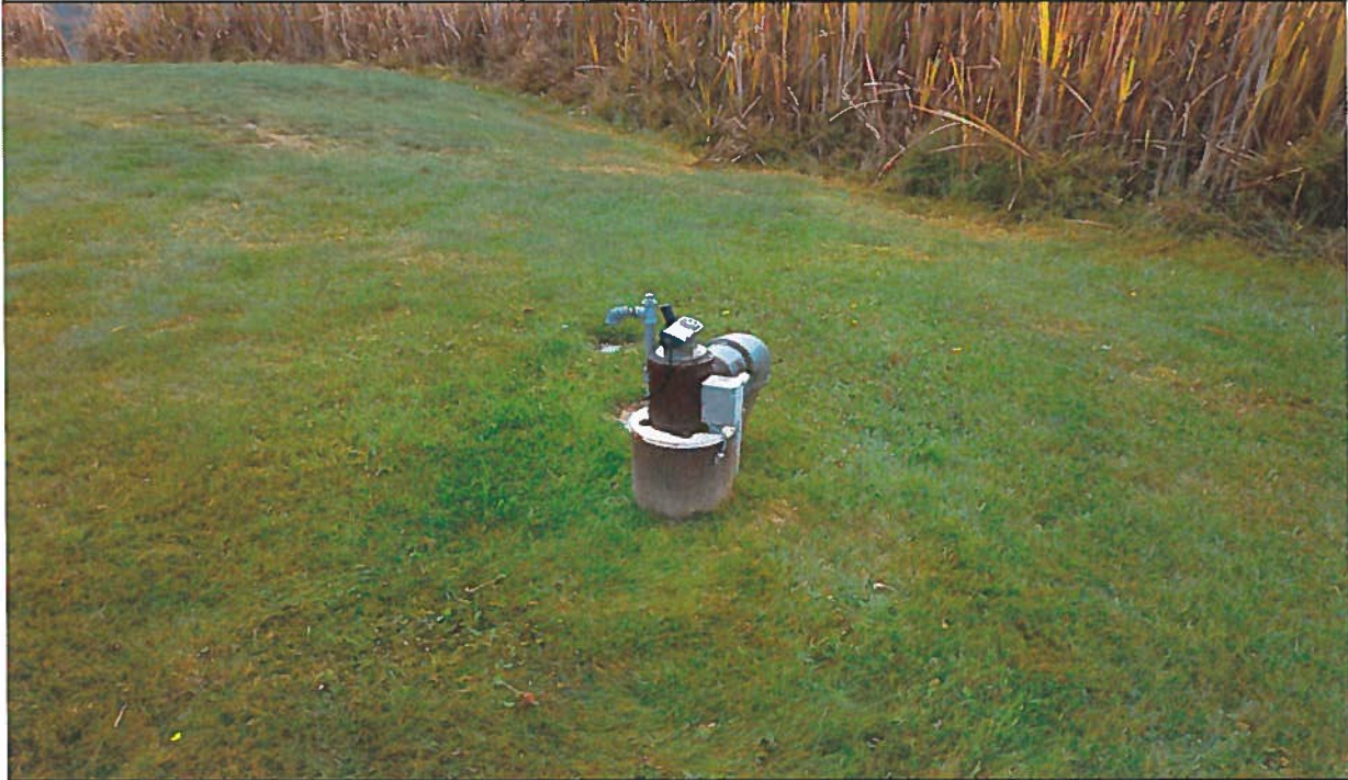
Point of Diversion: View of ground water well adjacent to and north of an irrigation/recreation storage pond located in the 'Cedars 9-Hole Golf Course'.
