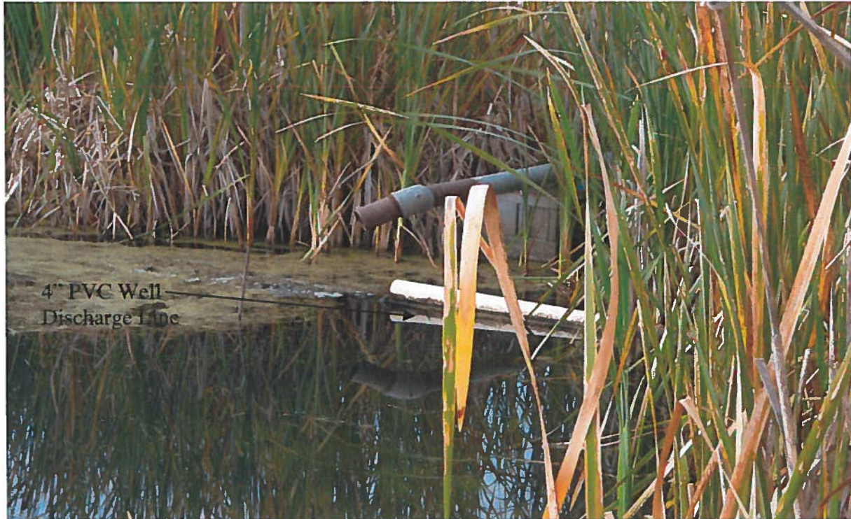
View westerly of the 4" PVC discharge line from the 'Cedars 9-Hole Golf Course' ground water well. The 4" steel pipe operates as a pressure relief mechanism for the golf course irrigation system.
