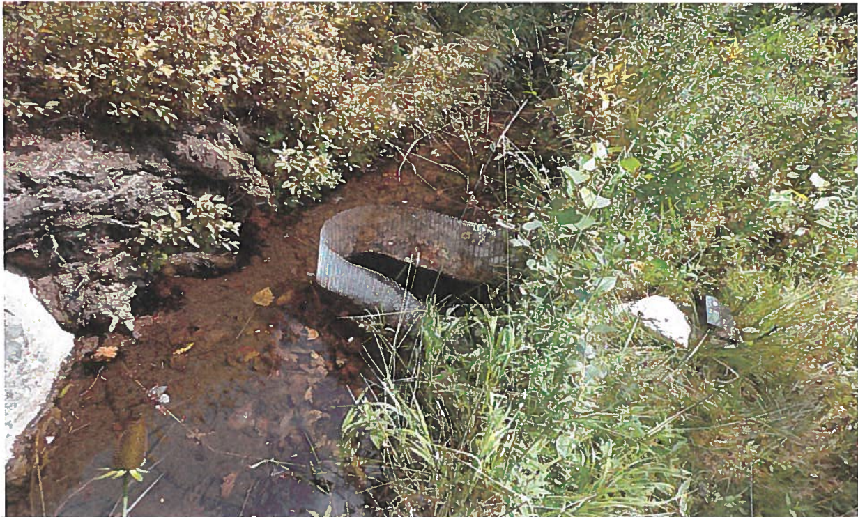
View southerly of the screened intake for the 4" PVC supply pipe which diverts water from the small irrigation ditch to discharge to the right holder's storage pond.
