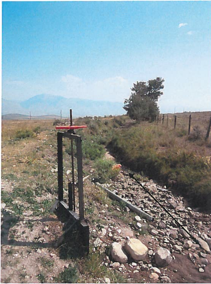
Headgate for Mill Creek water
