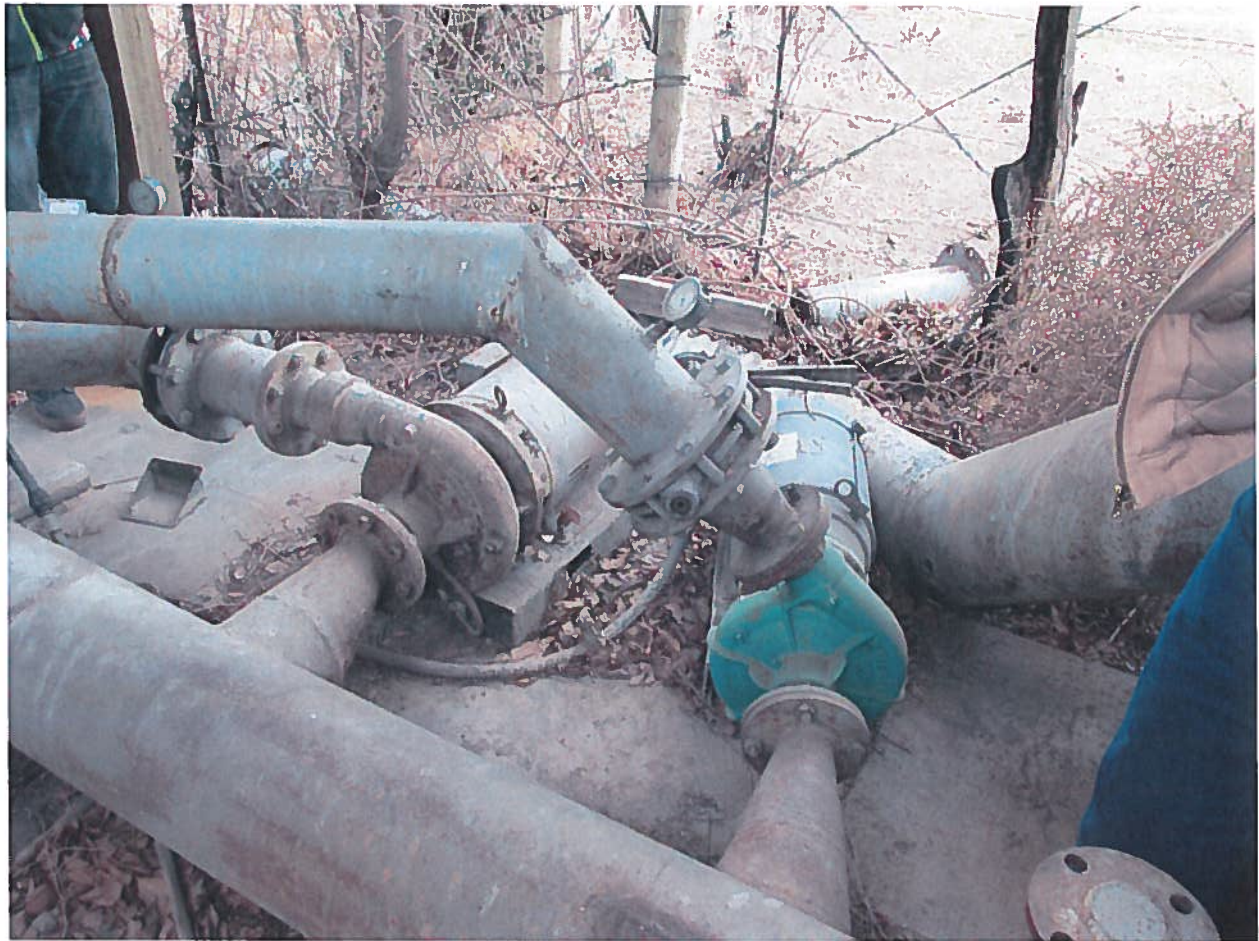
Pump house #1. Pump used for 61-7681 is green to the right. The pump house actually directs water to other places using irrigation from canal.
