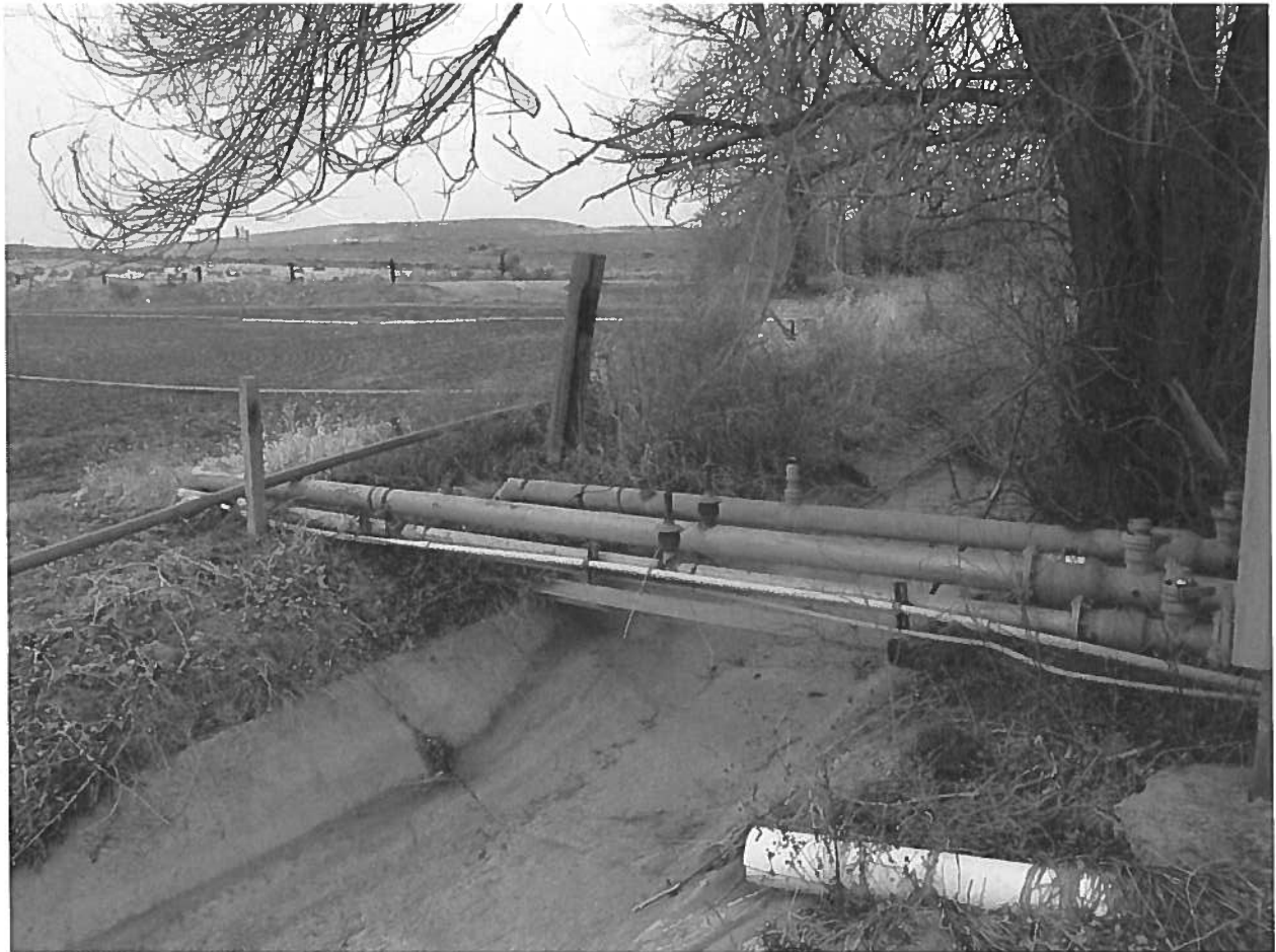
Water lines run from pump house (right) to different places of use. Water for irrigation moves under freeway and onto Farris property. Looking north from west side of pump house.
