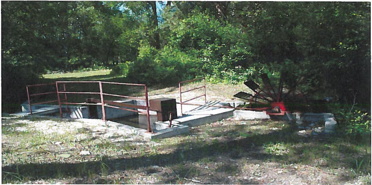
Fish screen upstream of pond
