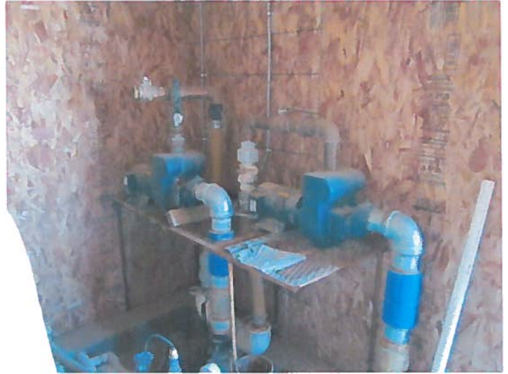
Booster pumps and piping
