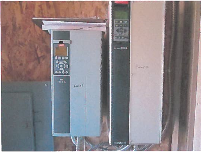
South Well Meters for Booster Pumps
