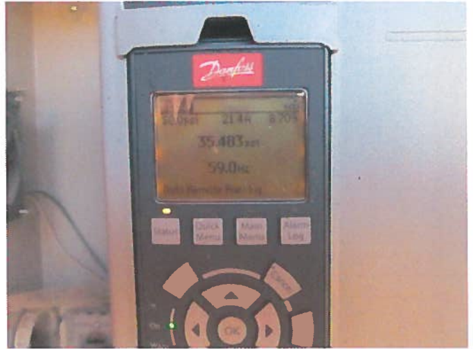
North Well meter
