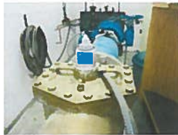
WELL #4 FLOW METER.JPG
