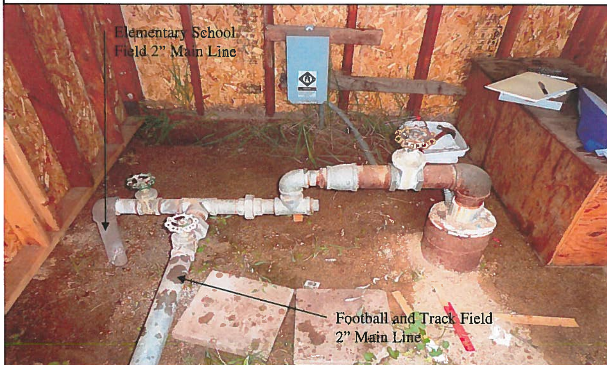
Point of Diversion: View inside the well and pump house of the ground water well and 3" and 2" galvanized steel discharge piping.
