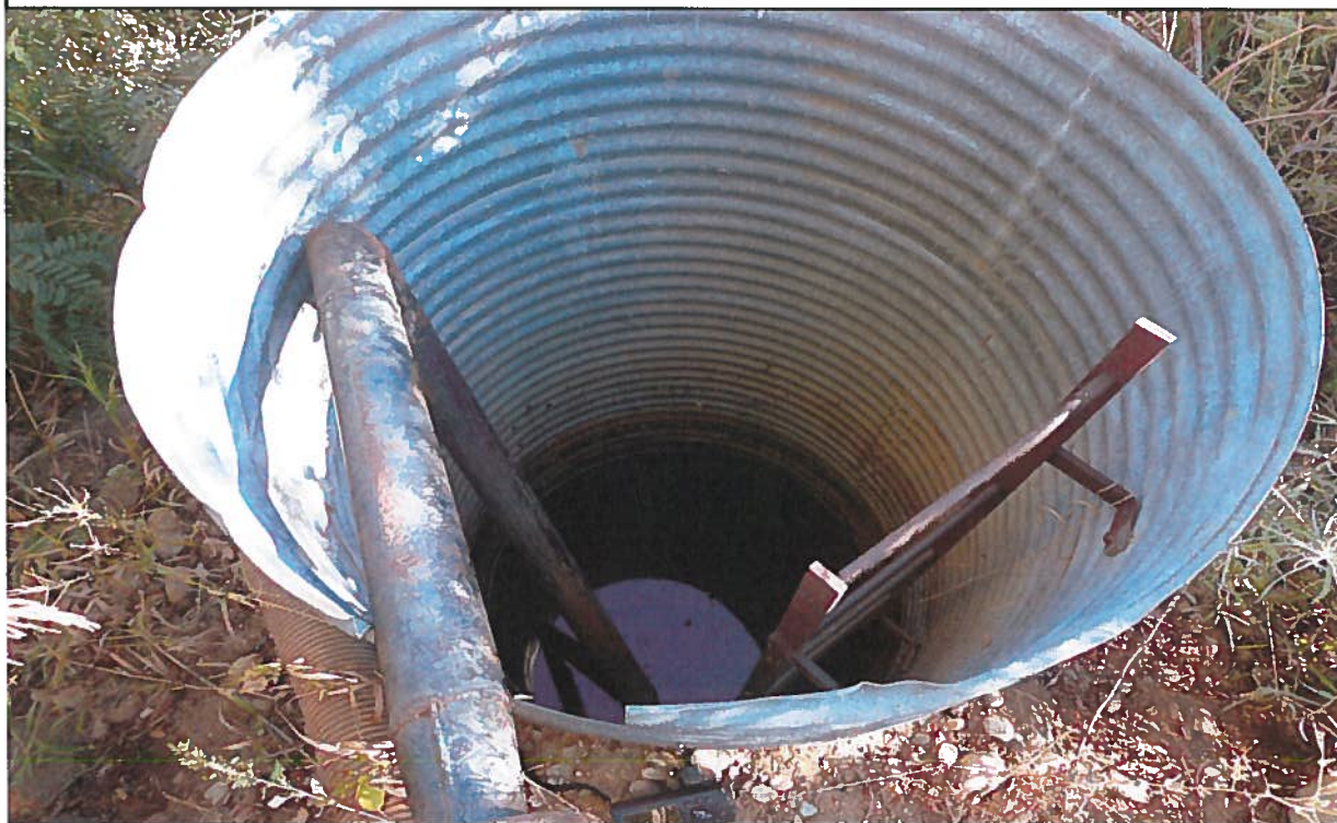
View of the 4' diameter x 10' deep CMP pumping sump. The 4" flexible hose suction line from Squaw Creek is shown to the left of the CMP pumping sump. A 10-hp pump diverts water from the CMP pumping sump sprinkler irrigation of fields.
