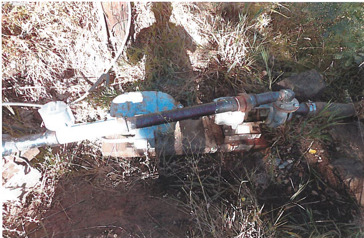
View of the pump and motor and the 4" PVC discharge line. Due to the low depth of Squaw Creek, the right holder is diverting water through the 4" flexible suction line to the pump, not from the 4' diameter CMP pumping sump.
