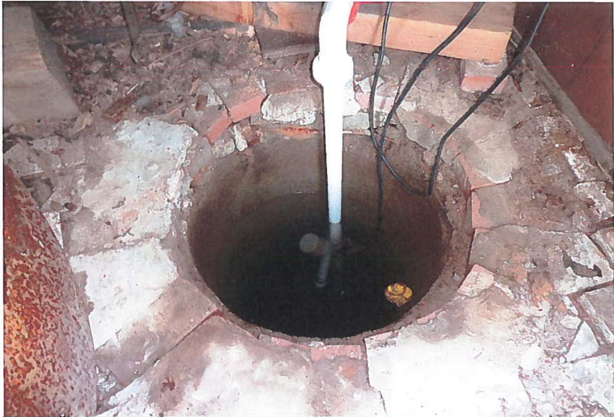
Point of Diversion: View of the 2' diameter concrete spring box and float switch.
