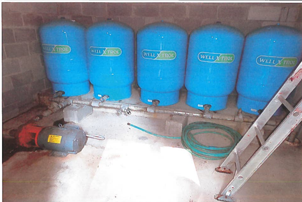
View inside of the pump house of the five (5) pressure tanks and the 1 1/4" galvanized steel supply line. A Berkeley 7.5-hp centrifugal booster pump is shown to the left.
