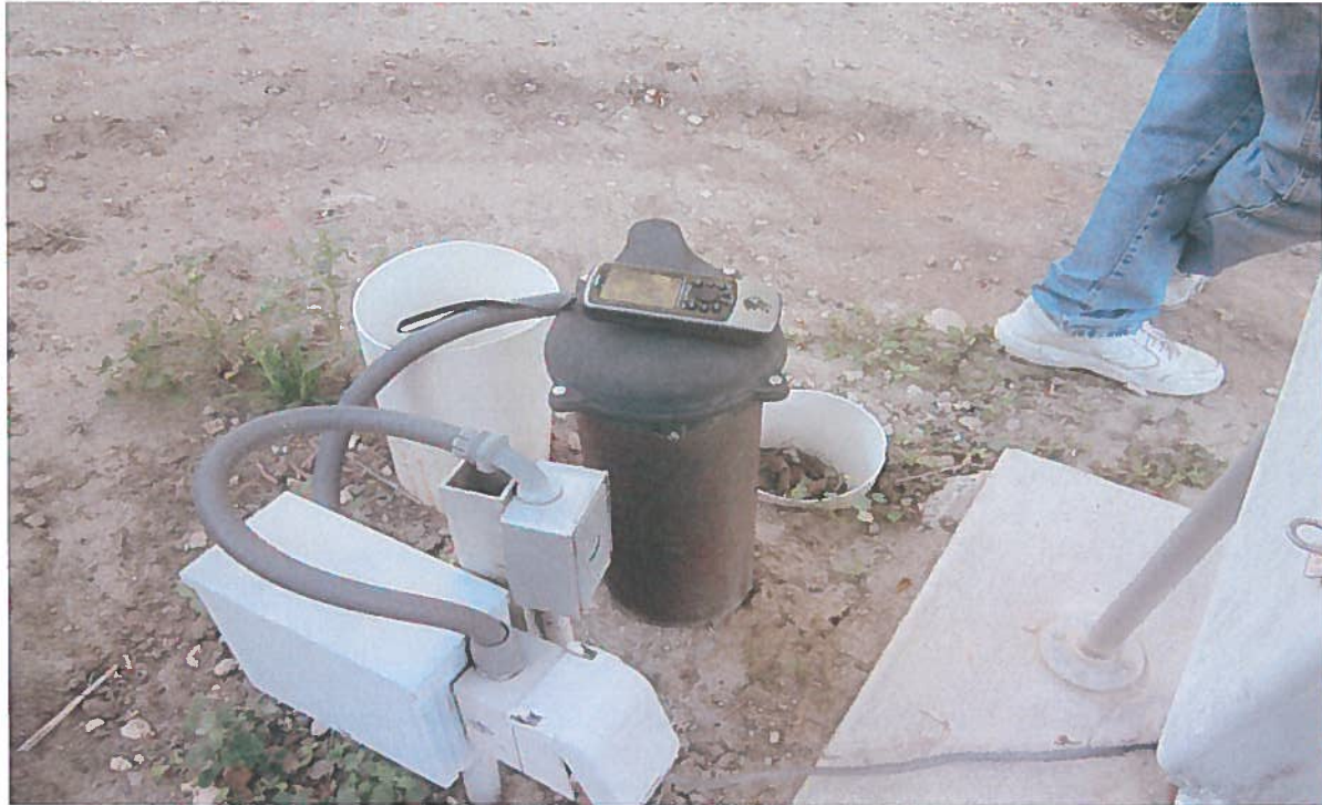
Well, 6" diameter, 3 hp submersible pump.
