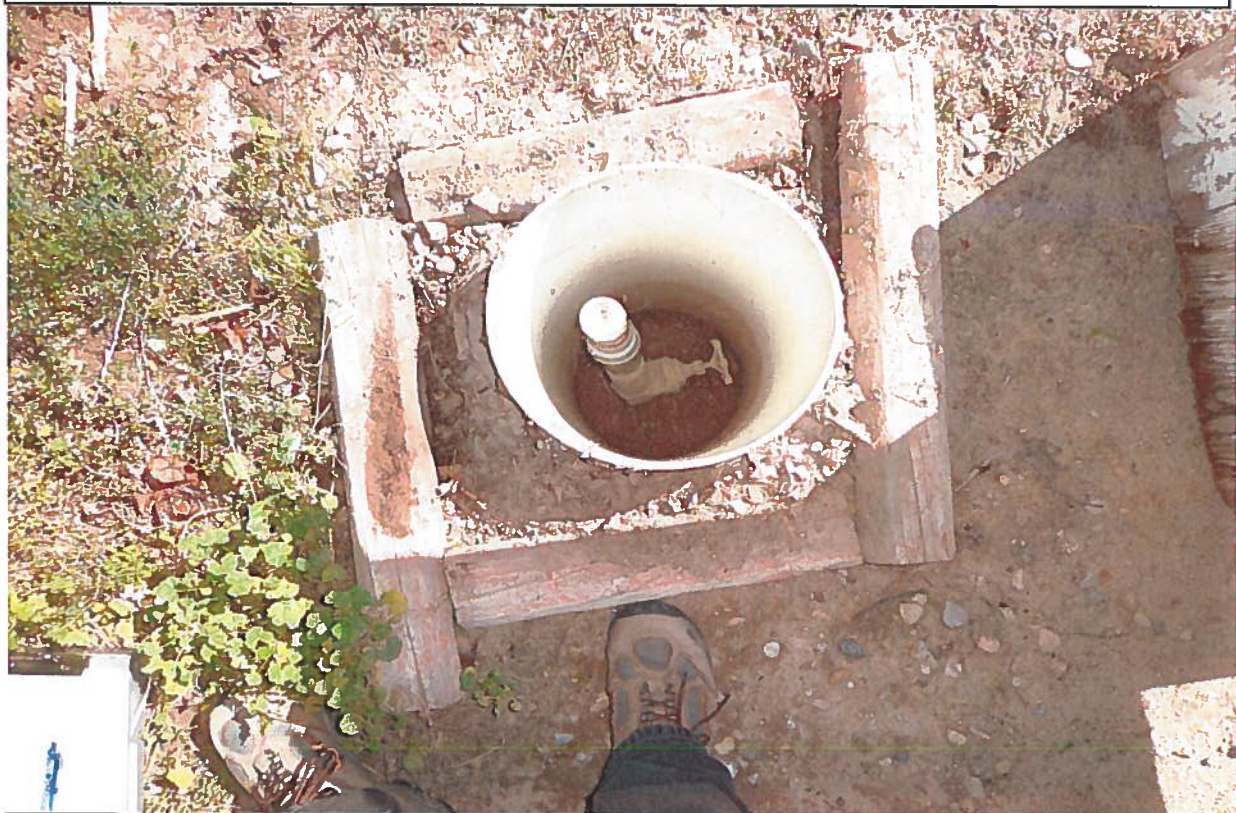
View of the typical fire protection 'flush ports'. A 2" galvanized steel riser reduces to 1 1/2" for fire hose connection. The development has two of the fire protection 'flush ports'.
