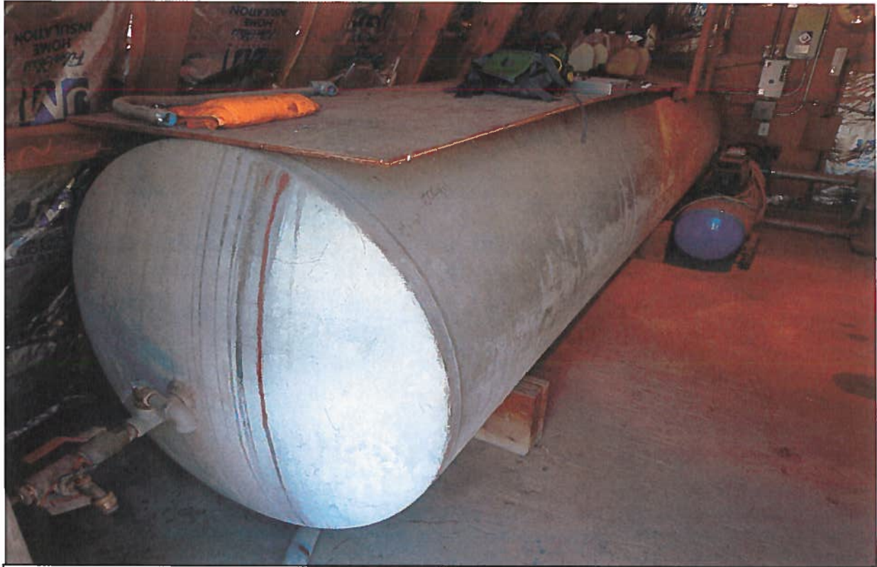
View inside the well and pump house of the 1,000-gallon steel pressure tank.
