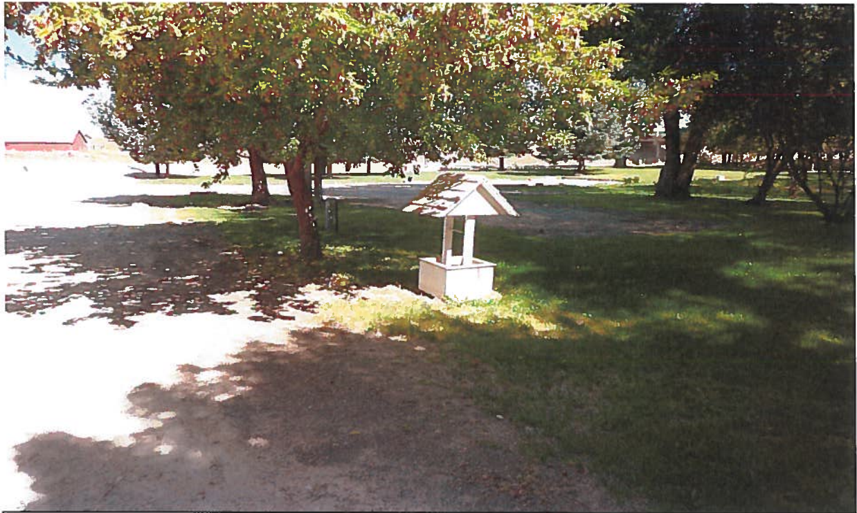
View northerly of the typical 'wishing well' which is placed atop the fire protection 'flush ports'.
