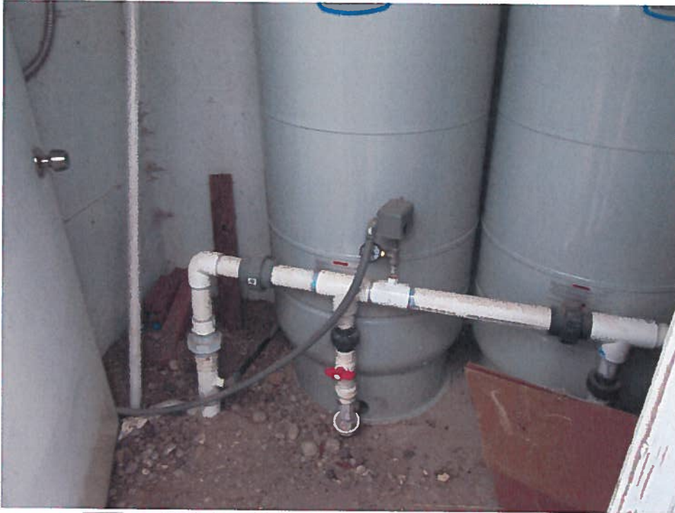
Pressure tanks and plumbing
