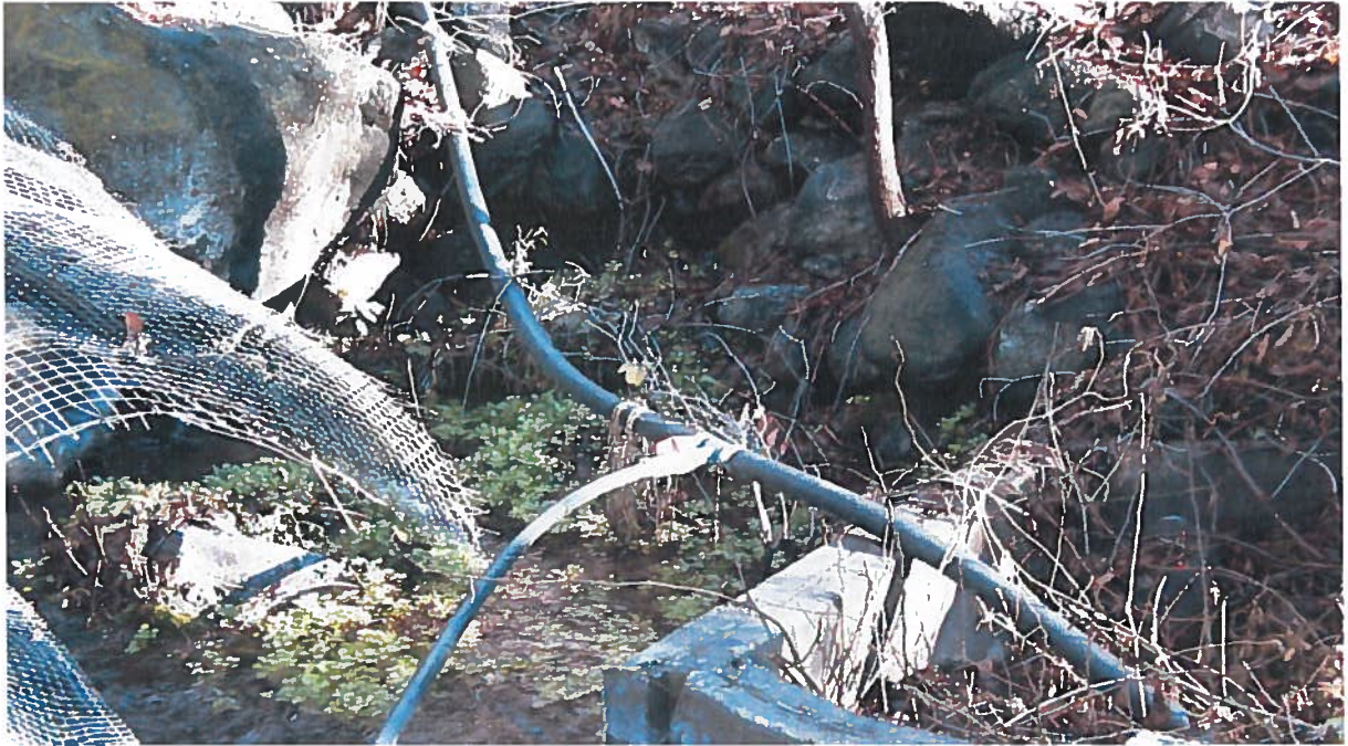
Service line branching off to home
