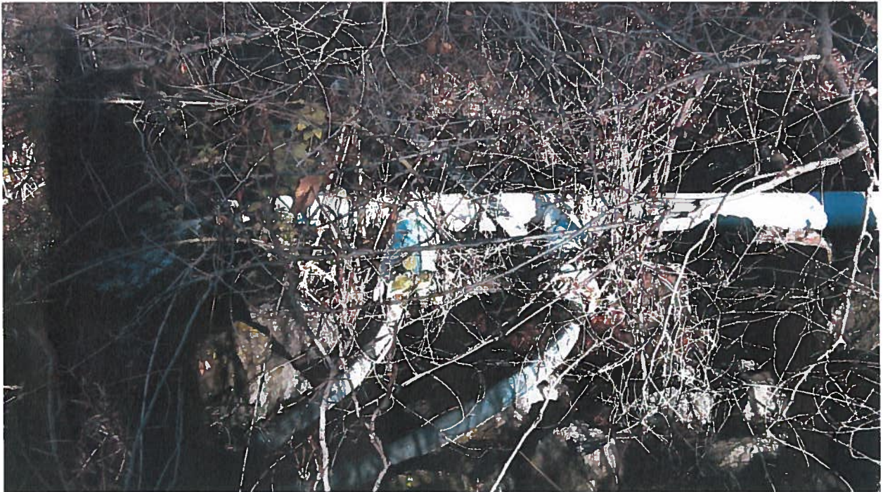
Flexible hoses branch off of six inch PVC pipe
