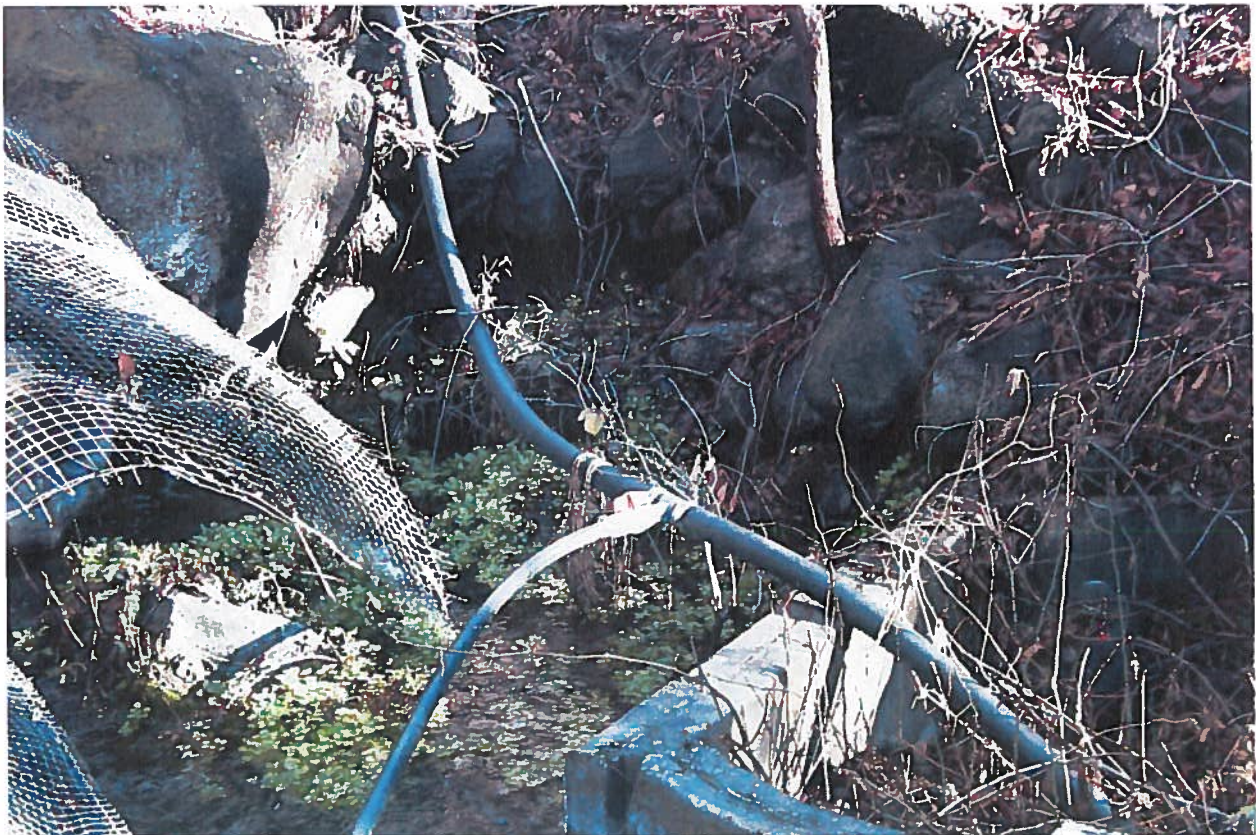
Water line to Tupper home
