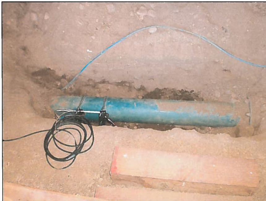
Figure 4: Flowmeter installation with well to photo right.
