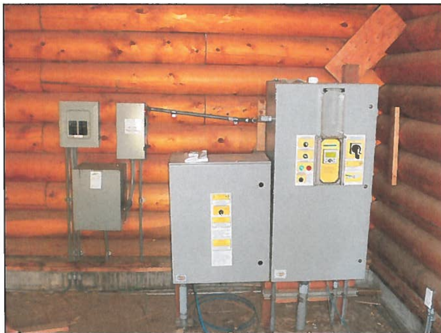
Figure 5: Well pump panel and VFD controller.
