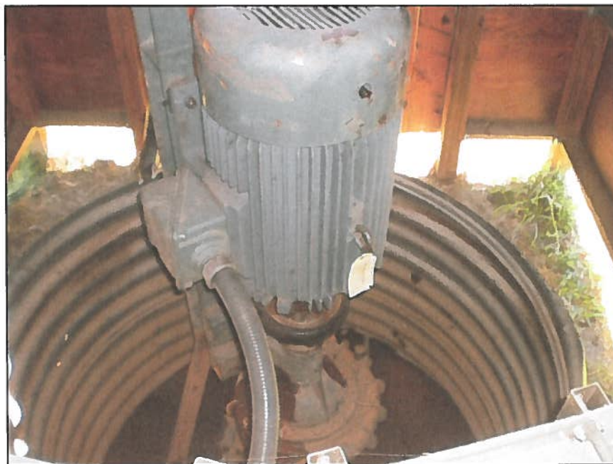
Figure 9: 100-hp secondary irrigation pump draws from pond 2.
