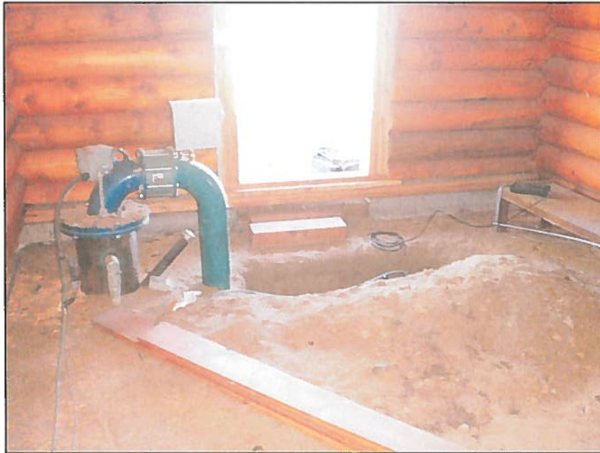
Figure 3: Irrigation well equipped with submersible pump. Well tag D0038988.
