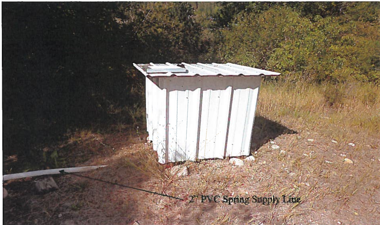
Point of Diversion: View northwesterly of the metal structure for an 18" PVC spring box.
