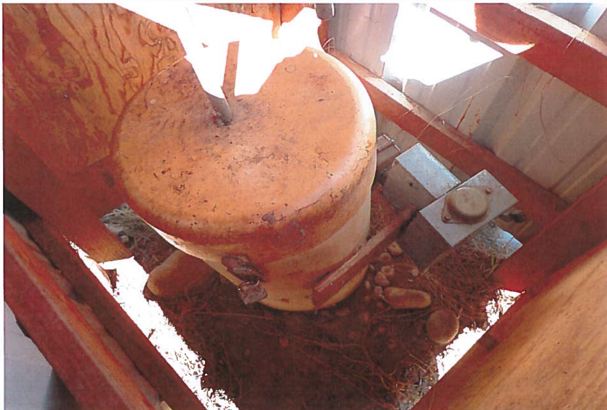
View of the 18" PVC spring box inside the metal structure. The spring box extends 15' below ground. A 2" PVC supply line, which penetrates a nearby hillside, diverts water from a spring to the spring box. A 1" PVC discharge line conveys spring water to a 1 1/4" PVC manifold located in the 12" PVC pumping stand pipe. A 4" PVC overflow pipe discharges overflow spring water to the Middle Fork of the Payette River.
