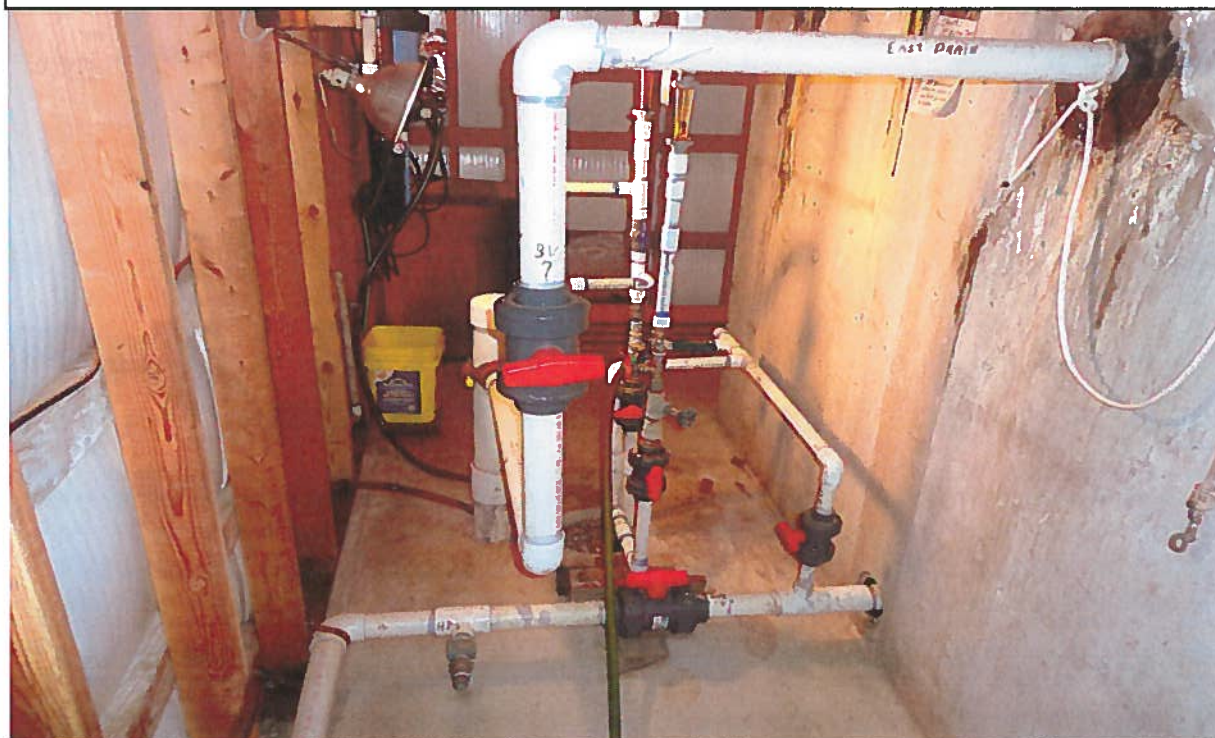
View of the 1" PVC supply line to the slow sand filter tank located inside the water treatment and water system control building.
