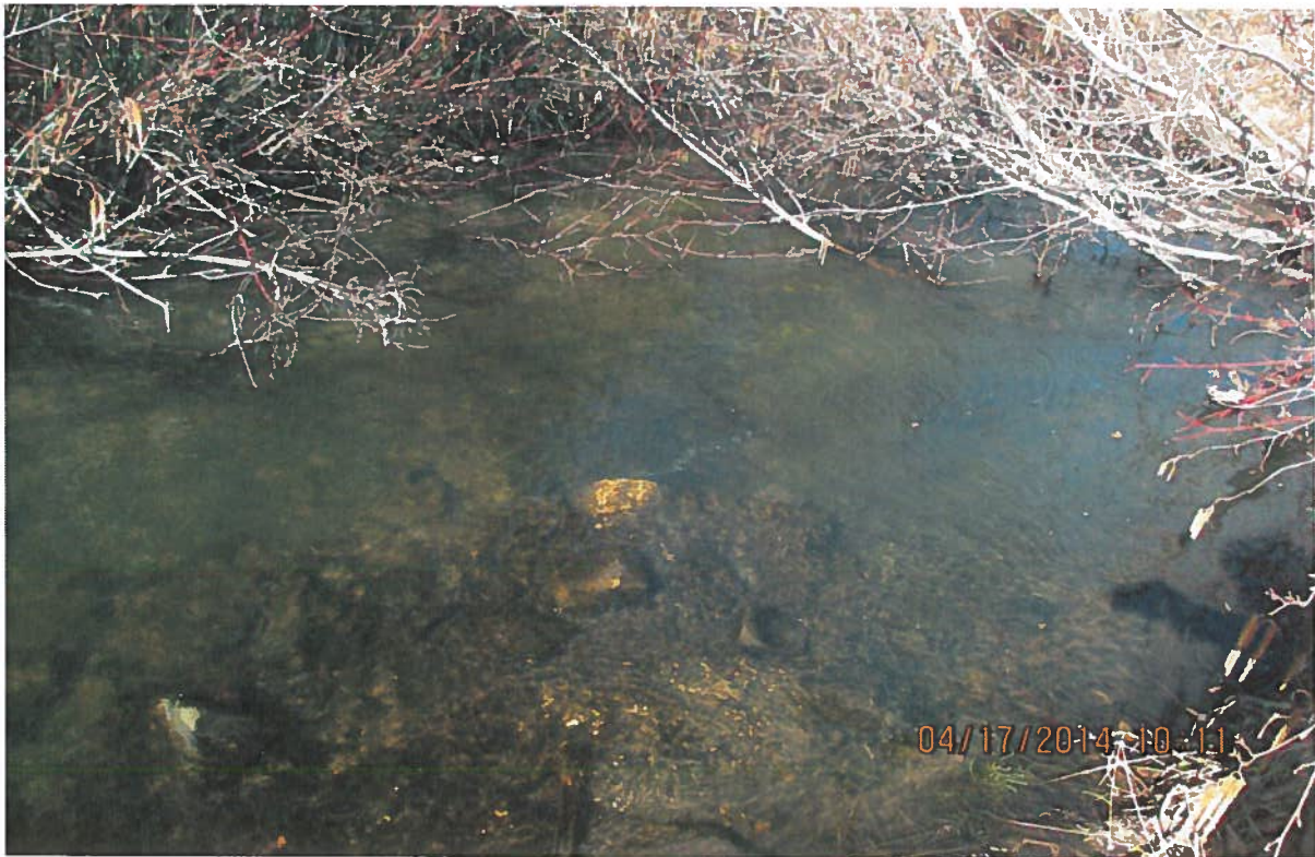
-113.588706, 44.946419: 10" return flow pipe, with broken butterfly gate
