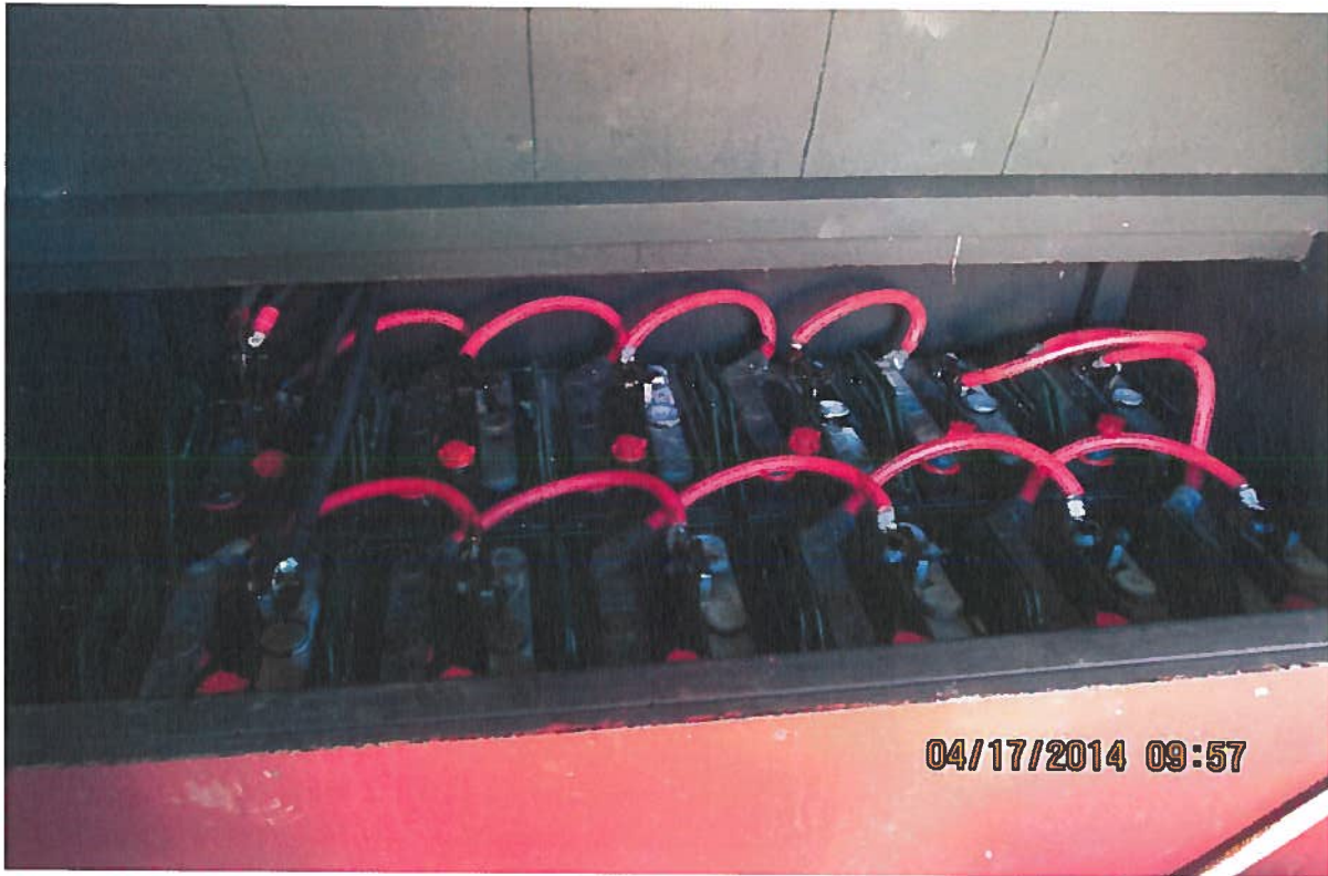
Battery Pack: 6, 2 volt batteries
