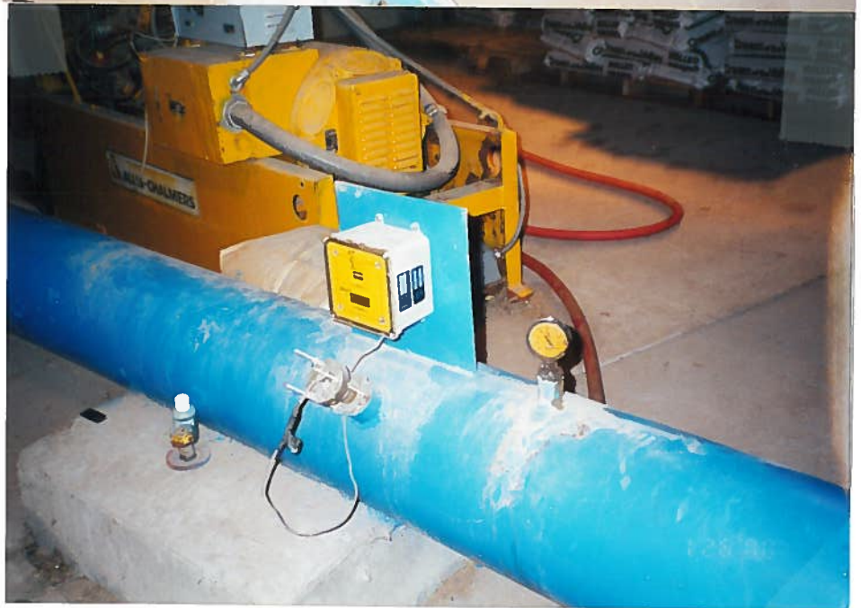
OLD flow meter (replaced 2001)
